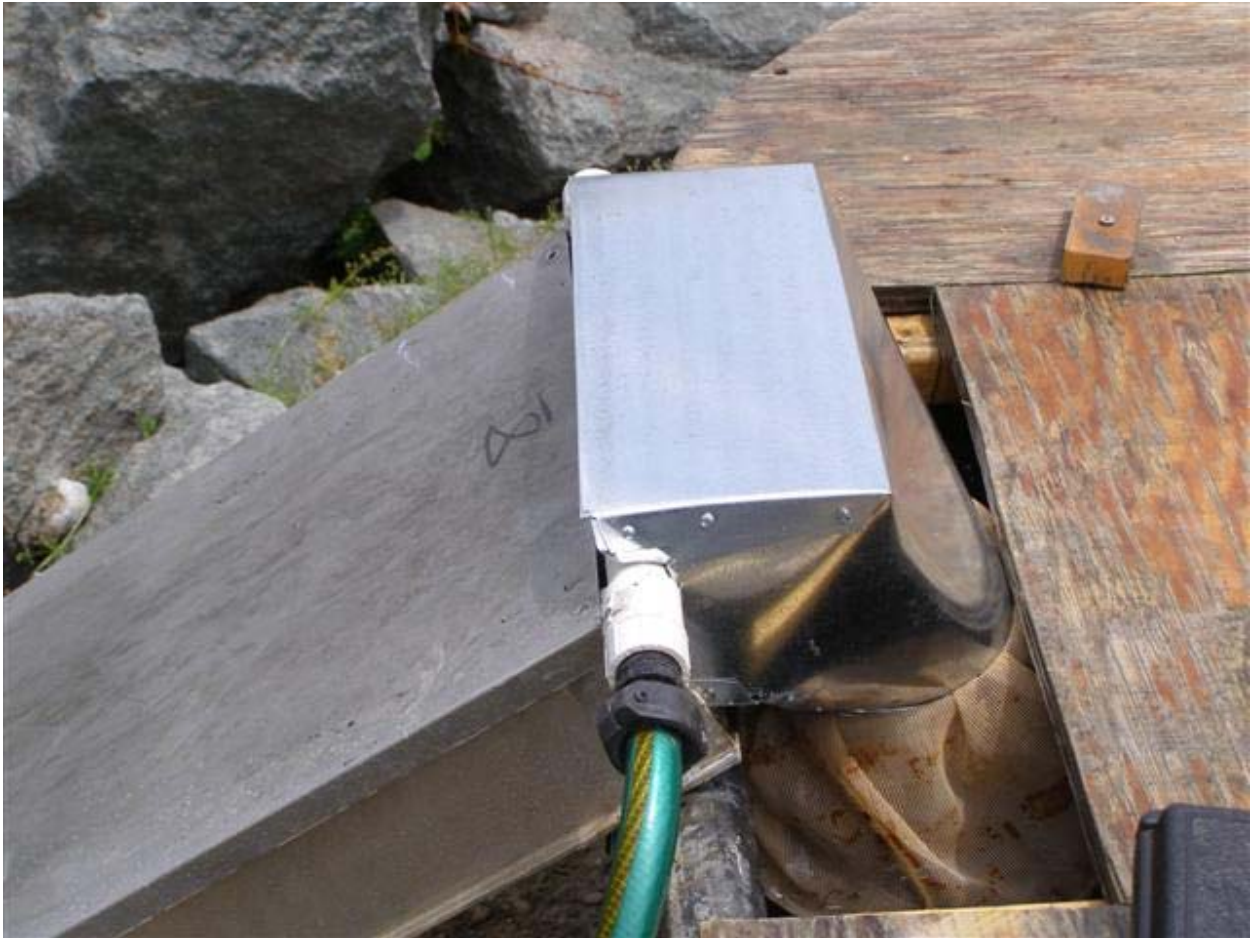
Figure 3. The cable tray emptying into a collection bag in a holding tank.
