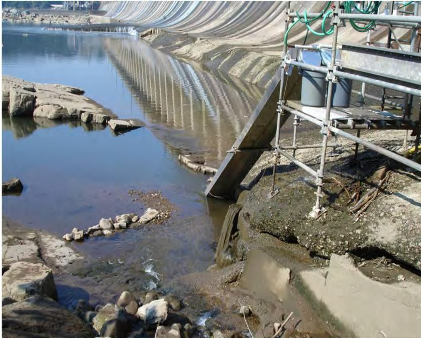
FIGURE 4.3-5: EAST RAMP WITH NATURAL ATTRACTION FLOW FROM INTERMITTENT STREAM, 2011.
