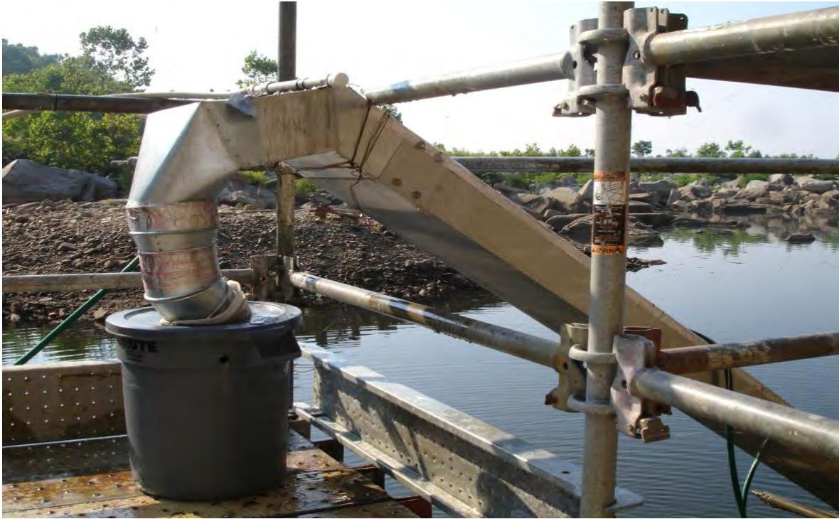
FIGURE 3-6: EAST SIDE ELVER RAMP COLLECTION TANK.
