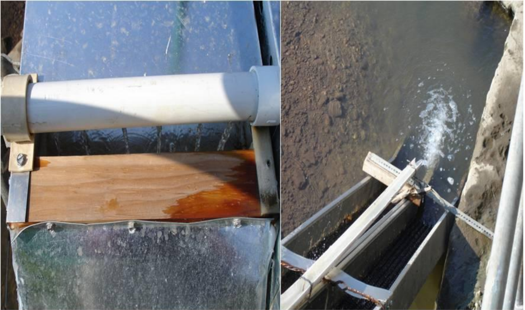
FIGURE 2-9: PHOTO OF SPRAY BAR AND ADDITIONAL FLOW.
