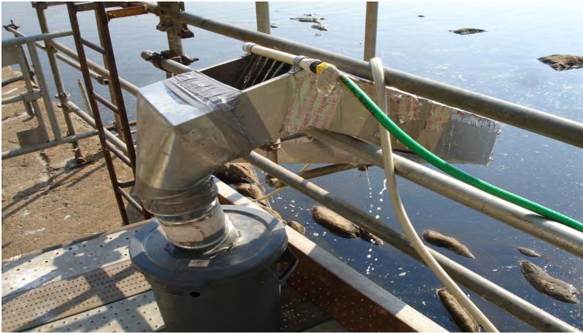
FIGURE 3-7: WEST SIDE ELVER RAMP COLLECTION TANK.
