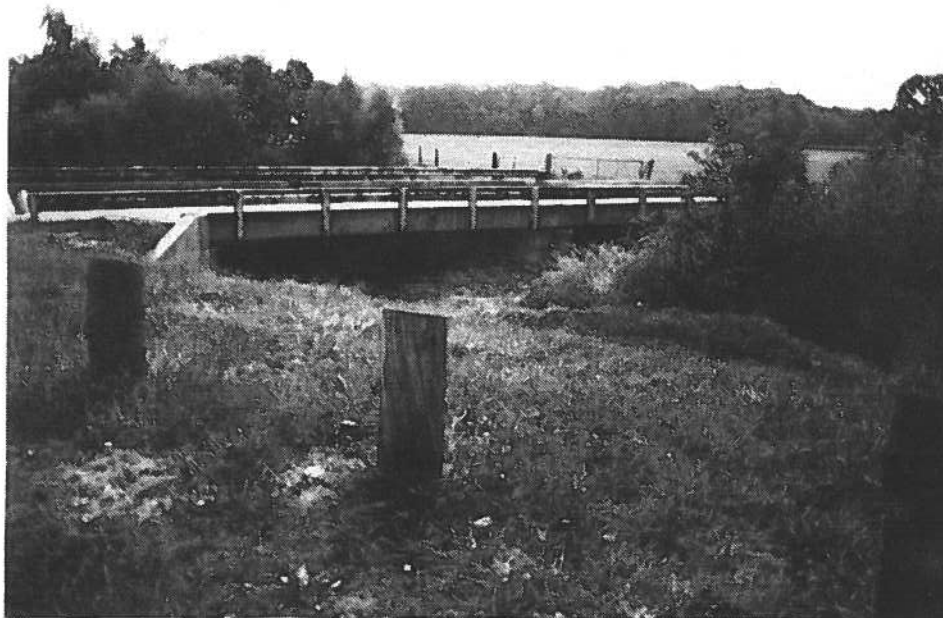
The Bethel Road bridge from the upstream side. The flow diverted near the Mountaindale Bridge will begin to rejoin Fishing Creek approximately 2,000 feet upstream of this bridge and continue this merge for another 1,000 feet downstream. Notice the flat terrain past the far bank where this junction of flow will occur.
