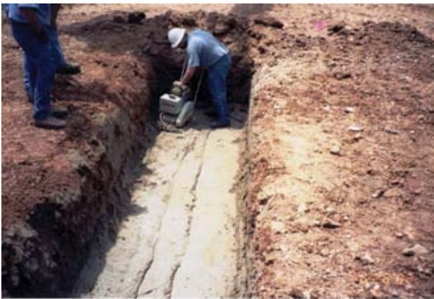
(c) Step 1 in constructing filter diaphragm. Trench has been excavated below grade at location of principal spillway conduit, and sand filter is being compacted in the trench. Conduit will be laid on top of trench after it is filled with filter material compacted to the required degree excavated and backfilled with sand.
