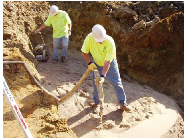
(d) Adding water to sand in filter diaphragm excavated below grade of principal spillway conduit prior to compacting
