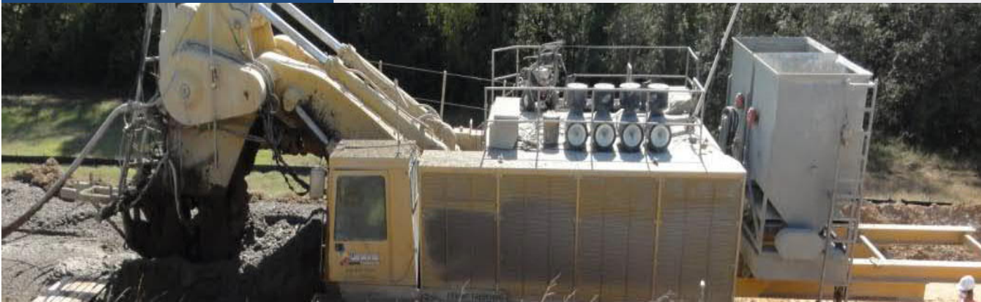
Grout Batch Plant
