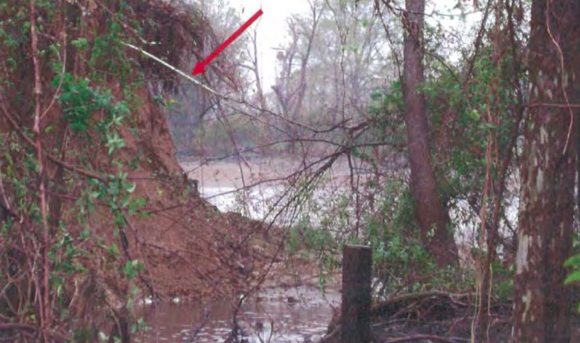
Edgewood Old City Lake Dam, TX Partial failure in 1988, failed in 2009 – both due to animal burrows Owner had removed 20-30 beaver in past few years
