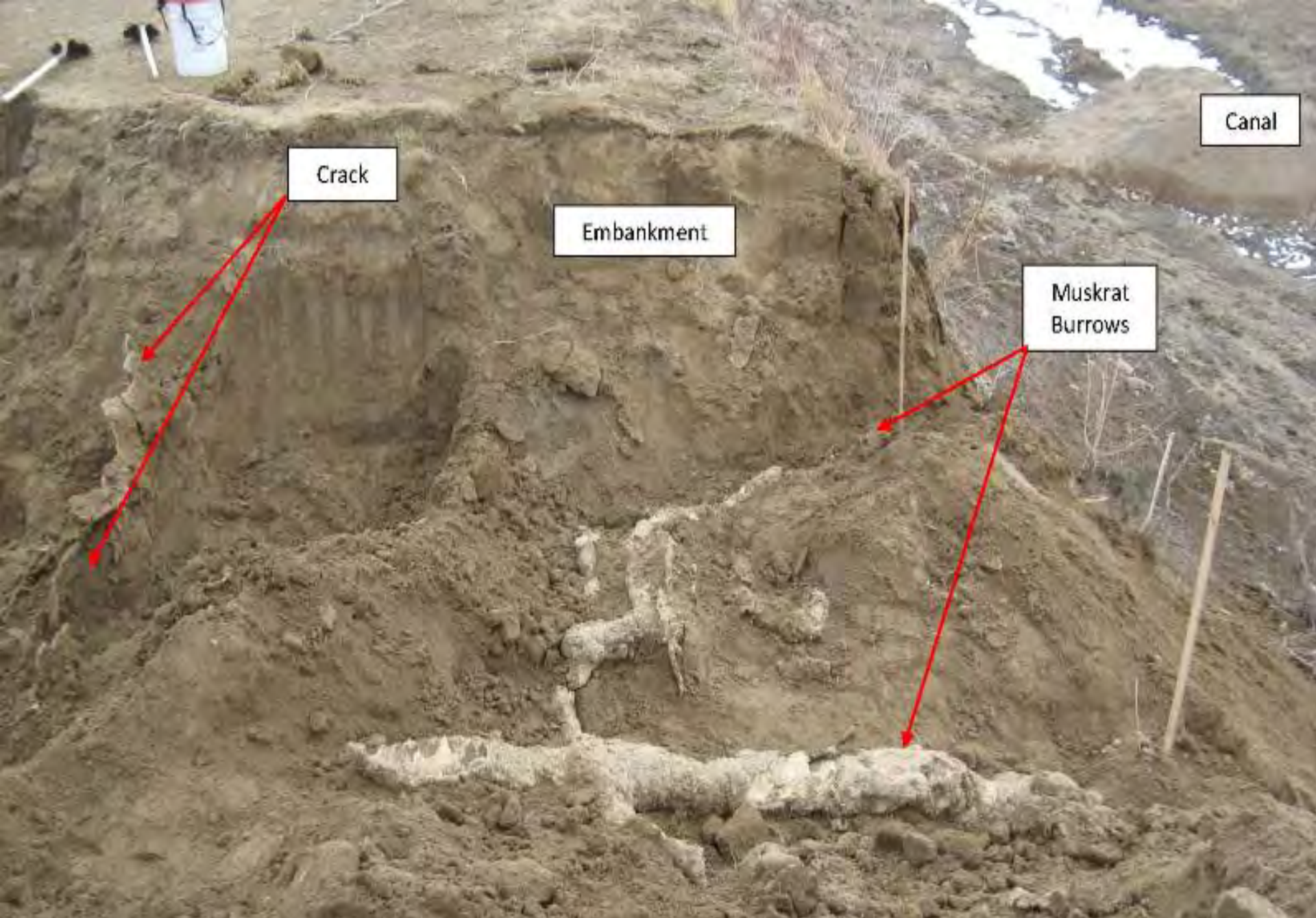
Truckee Canal Breach – Source: USBR Investigative Evaluation Report March 2008
