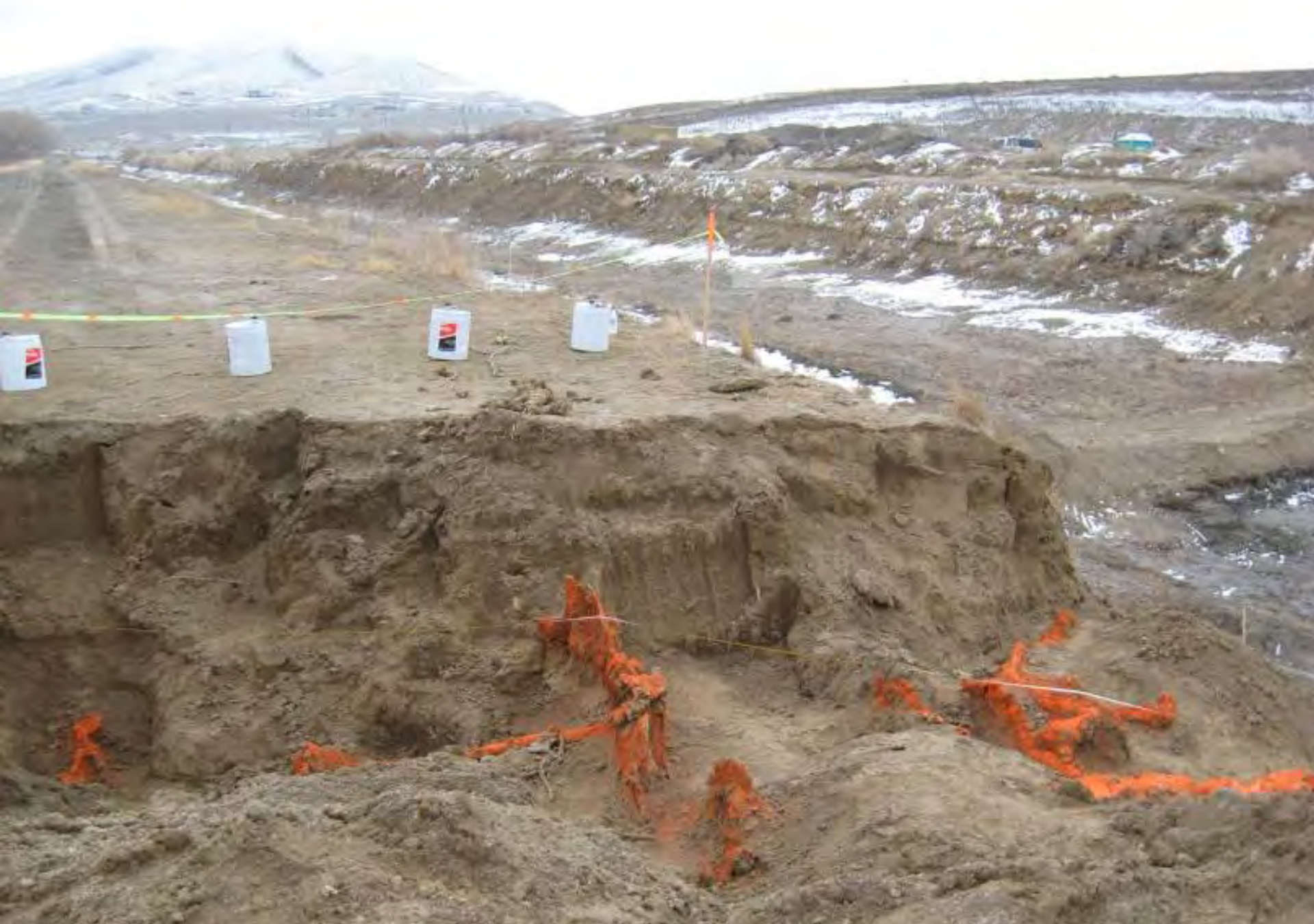
Truckee Canal Breach – Source: USBR Investigative Evaluation Report
