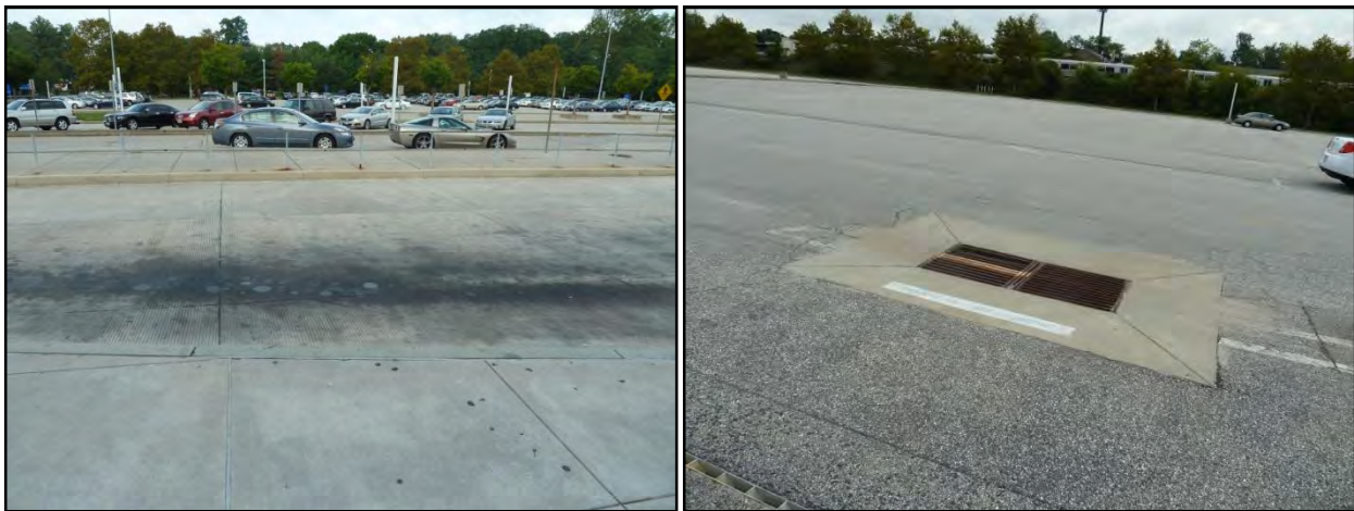
Figure 4-18: Staining at Bus Stop (left) and Impervious Surface (right) at HSI_C_0202
