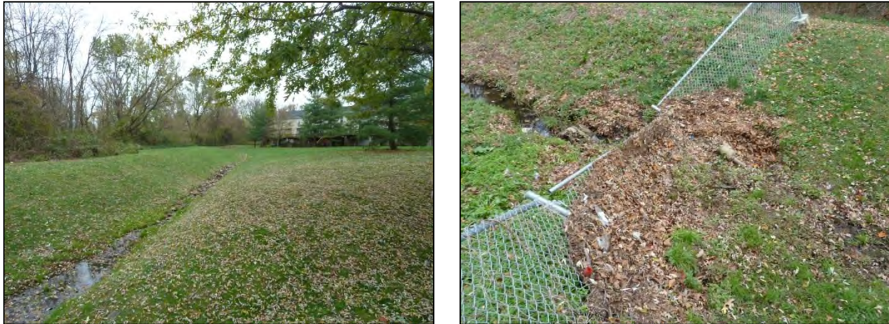
Figure 4-24: Channelized Grass Inflow (left) and Damaged Fence (right) at SWM_C_334
