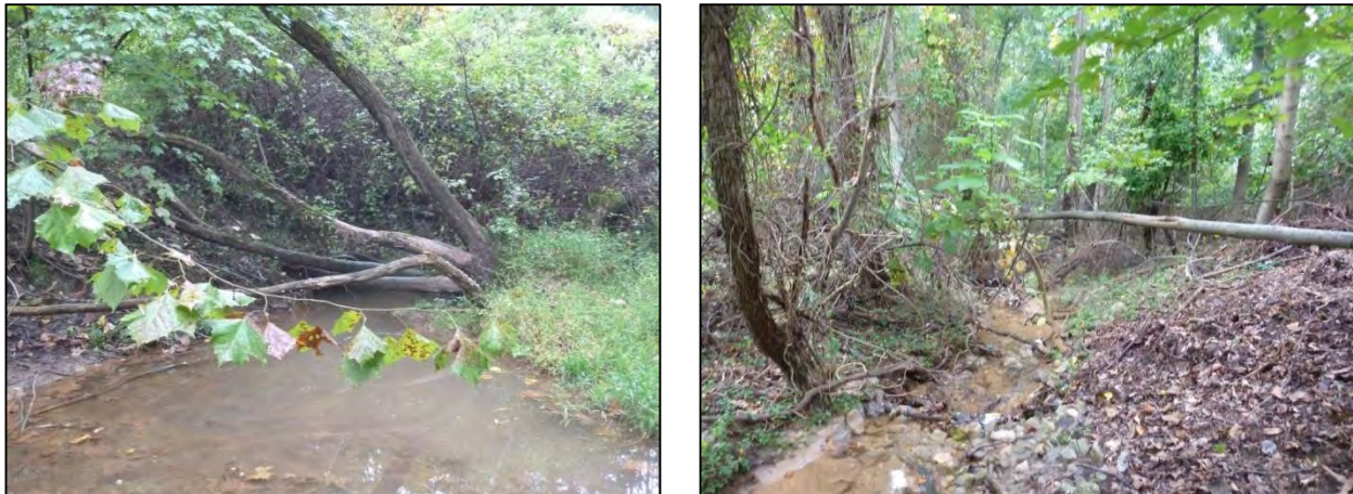
Figure-4-14: Down Tree Branches at Pond Outfall (left) and Low Flow Channel (right) at SWM_C_984
