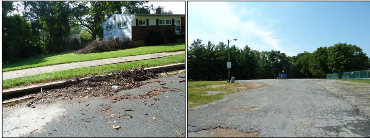
Figure 4-17: Street Sweeping at NSA_C_55 (left) and Potential Impervious Cover Removal or BMP practice at NSA_C_57 (right).
