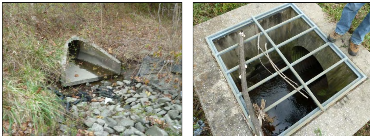
Figure-4-27: Undercutting and Erosion at Inflow Endsection (left) and Control Structure with Flowing Underdrains (right) at SWM_C_961
