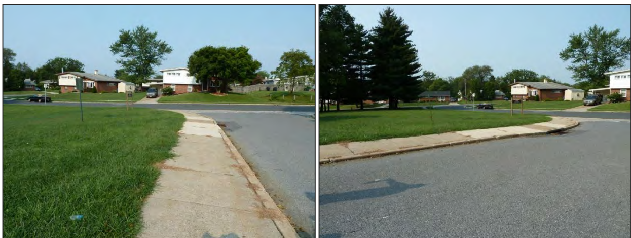
Figure 4-9: Potential Locations for Removal of Curb Inlets and Construction of Stormwater Retrofits at ISI_C_111
