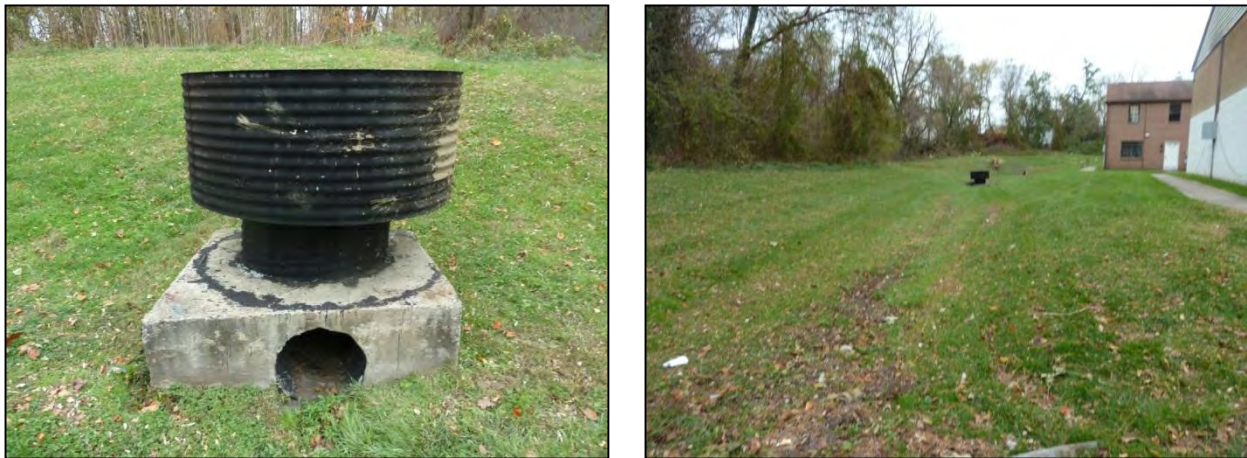
Figure 4-12: Riser with 18" Low Flow Pipe (left) and Grass Swale Leading to Riser (right) at SWM_C_715
