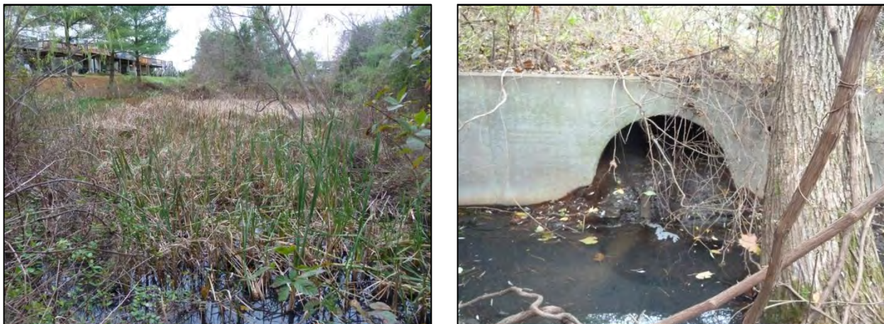
Figure-4-25: Invasive Species, Ponding (left) and Sediment Blocking the Downstream Outfall (right) at SWM_C_432
