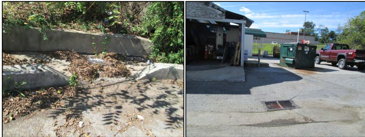
Figure 4-30: Evidence of Clogged Inlet and Leakage from Dumpster at HSI_C_0402
