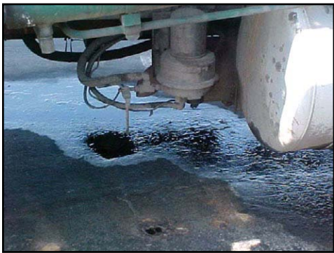
Figure 7. Equipment should receive routine preventative maintenance to prevent drips and leaks.
