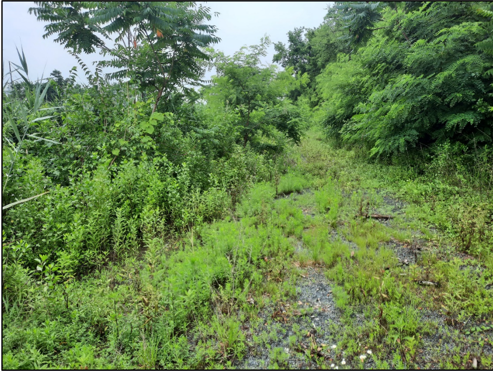
060619-5: Area originally cleared and regraded for the installation of underground utilities along the western edge of the Site.
