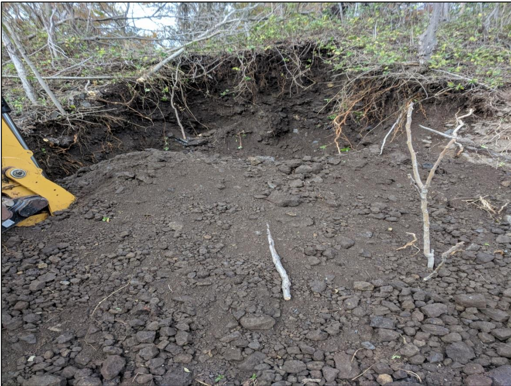
Photo 18: View of GRY-001-TP after excavation activities. Fine to coarse grained soils (silt, sand, and gravel) and slag fill materials were observed. A PID reading of 6.7 ppm was recorded.
