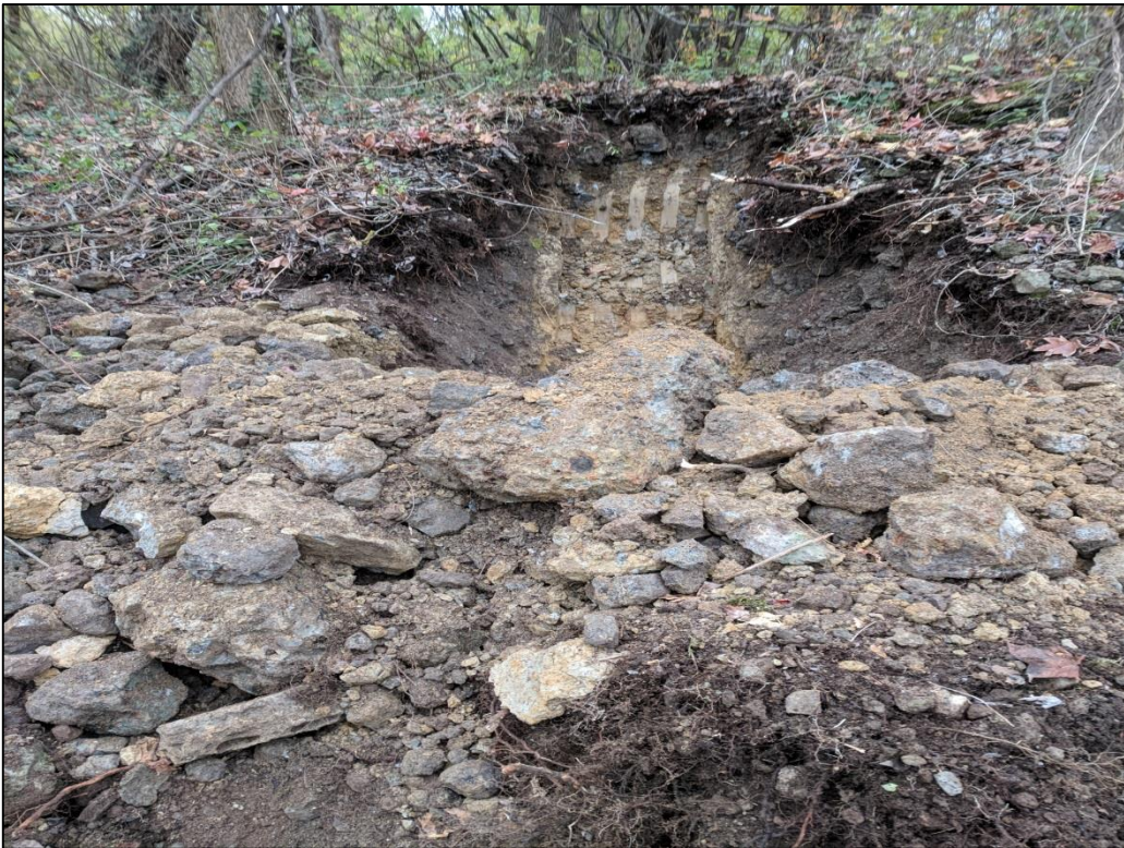
Photo 10: View of A5-005-TP after excavation activities. Fine to coarse grained soils (silt, sand, and gravel) and slag fill materials were observed. A PID reading of 20.0 ppm was recorded.
