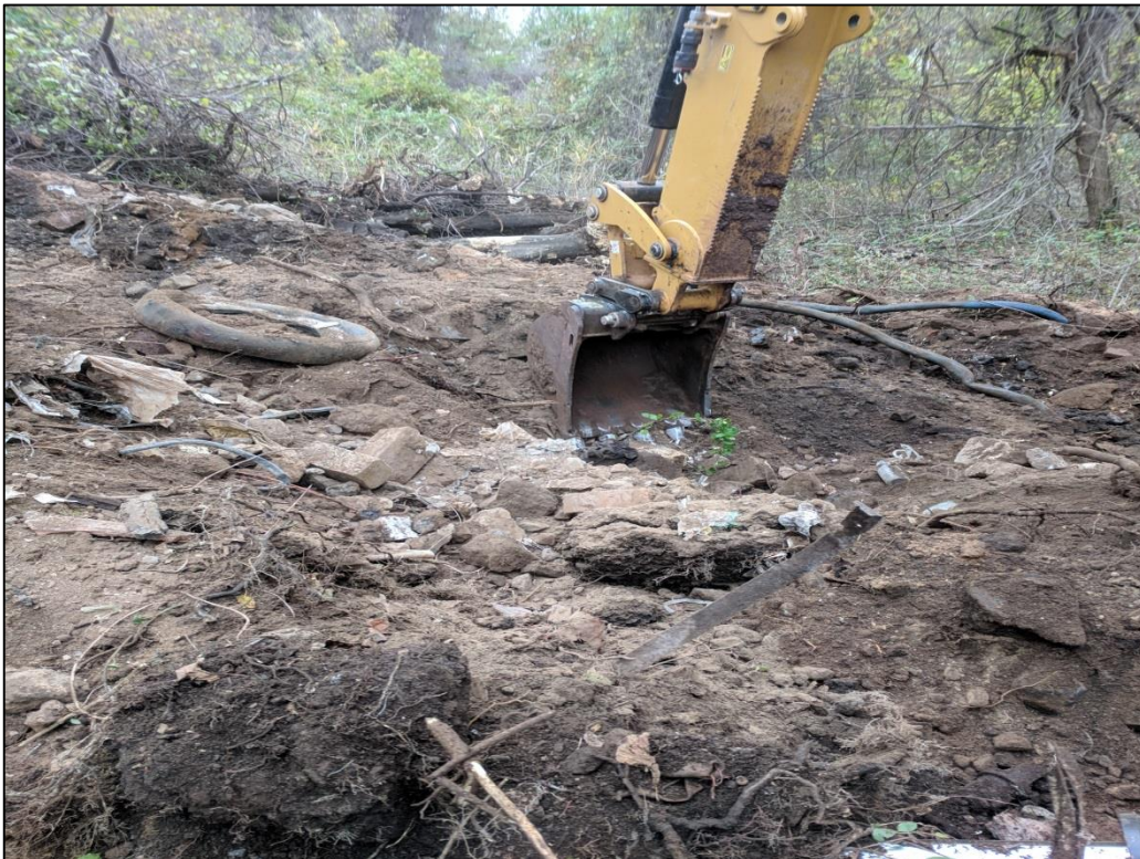
Photo 2: View of A5-001-TP during excavation activities. Trash and fine to coarse grained soils (silt and sand) and slag fill materials were observed. PID reading of 1.4 ppm was recorded.
