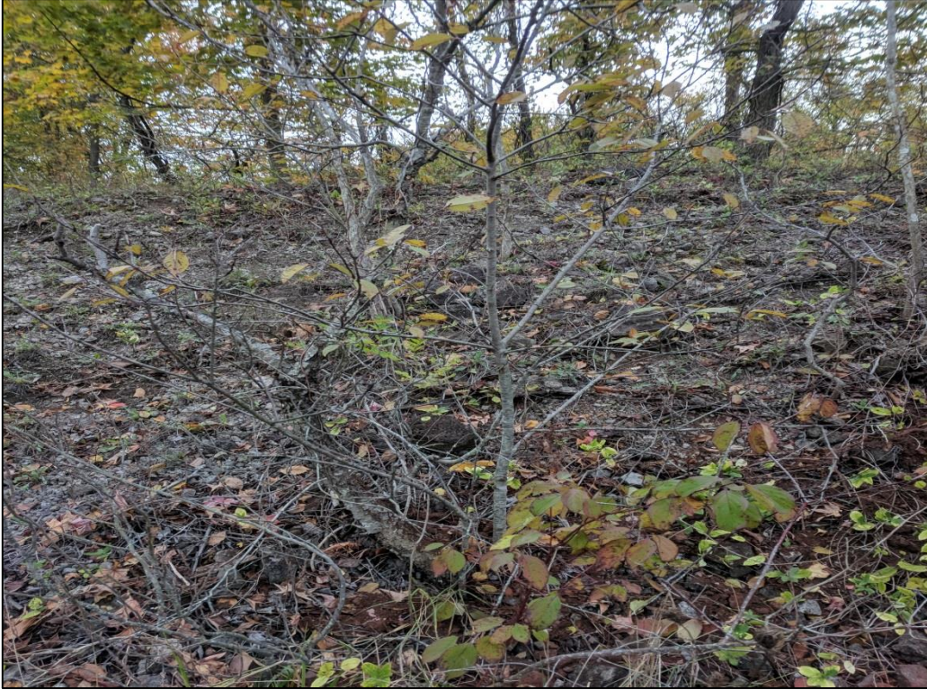
Photo 11: View of A5-006-TP prior to excavation activities. View is from the bottom of the berm.
