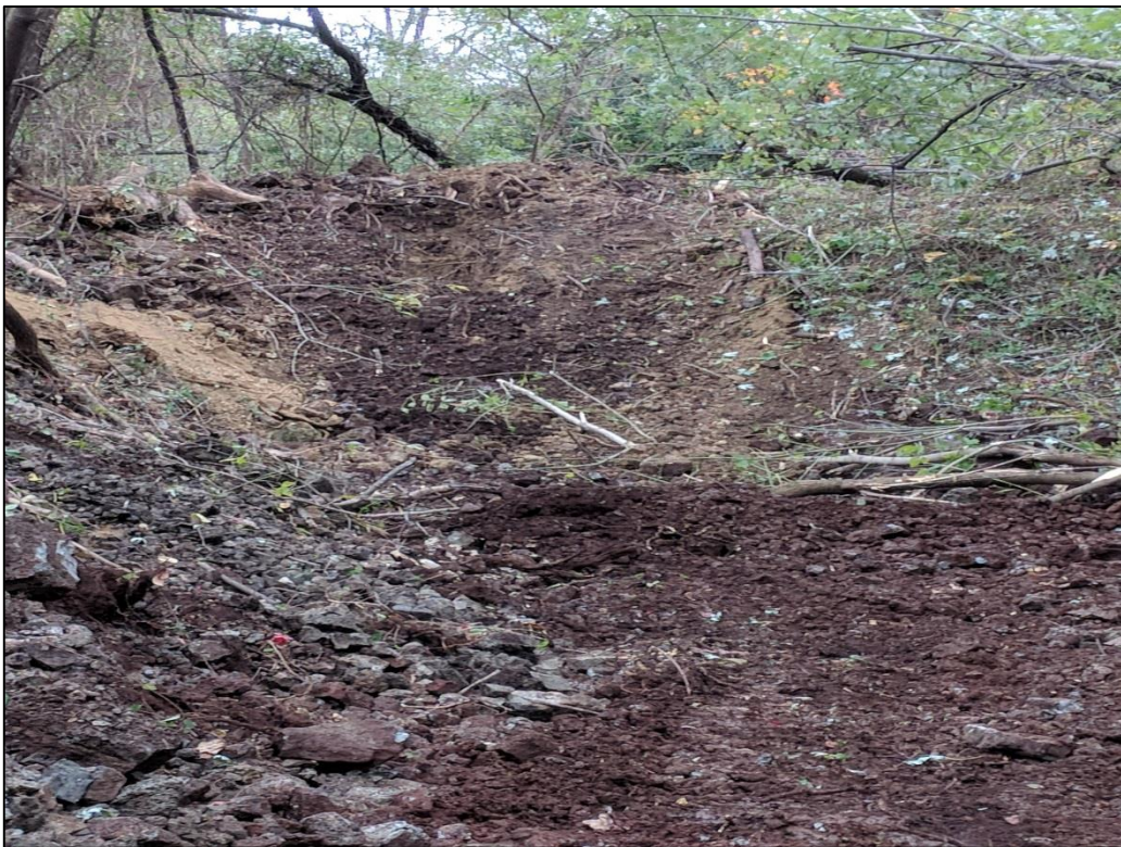
Photo 14: View of A5-007-TP after excavation activities. Fine to coarse grained soils (silt, sand, and gravel) and slag fill materials were observed. PID reading of 2.8 ppm was recorded.
