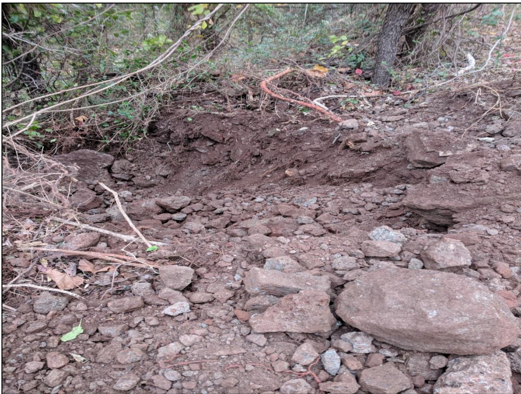
Photo 8: View of A5-004-TP after excavation activities. Fine to coarse grained soils (silt, sand, and gravel) and slag fill materials were observed. PID reading of 4.1 ppm was recorded.
