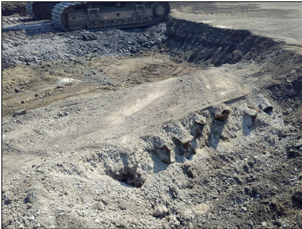
07/16/19-4: View of the railway structure in the northern section of the excavation.
