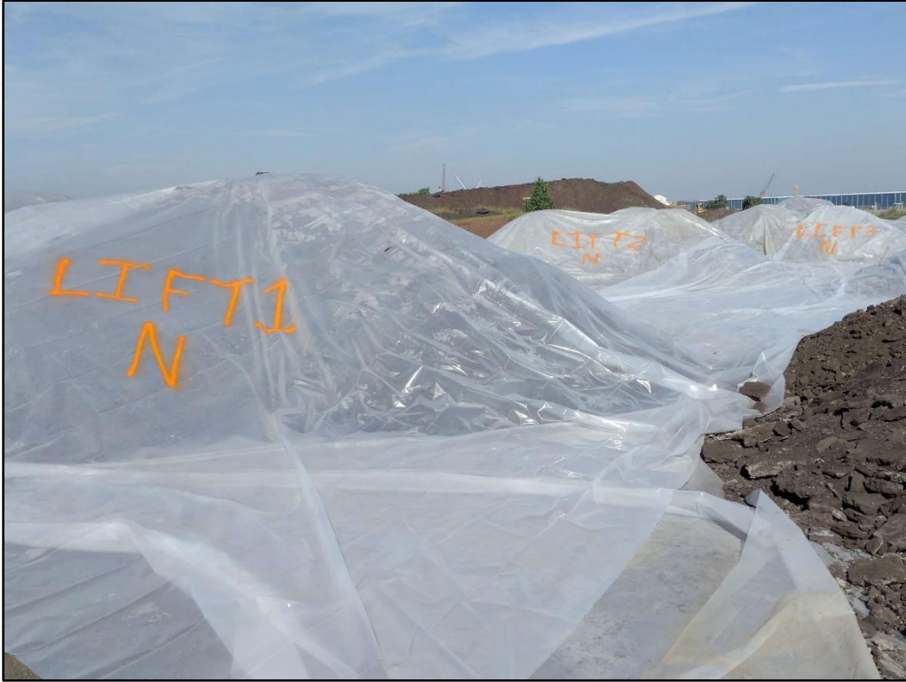
07/16/19-7: View of the covered and labeled stockpiles. The stockpiles are labelled on multiple sides for clear identification of each lift and excavation section.
