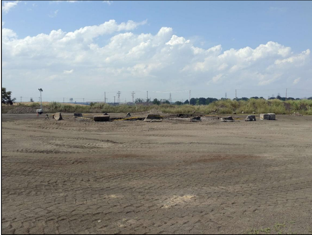
07/17/19-2: View to the north of the concrete barrier marked with yellow caution tape surrounding the completed excavation.
