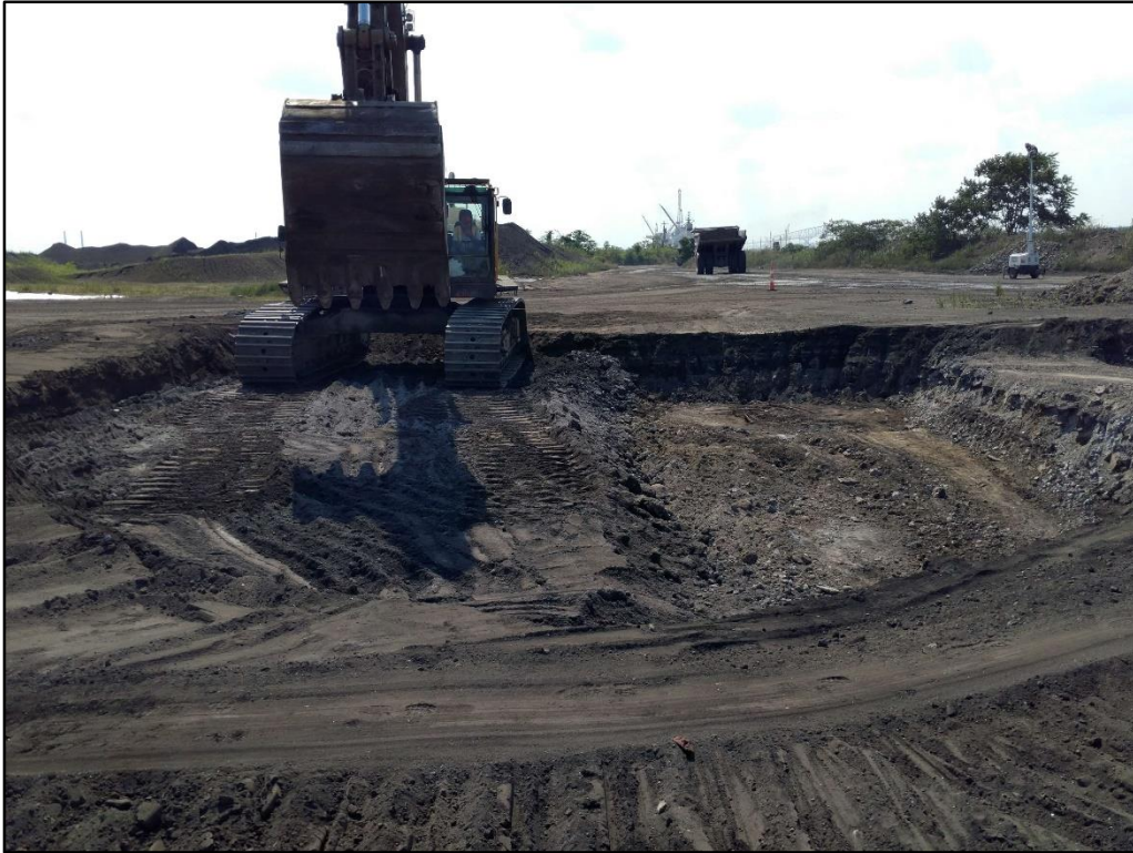
07/16/19-5: View to the west of the excavation at the end of the first day of digging.
