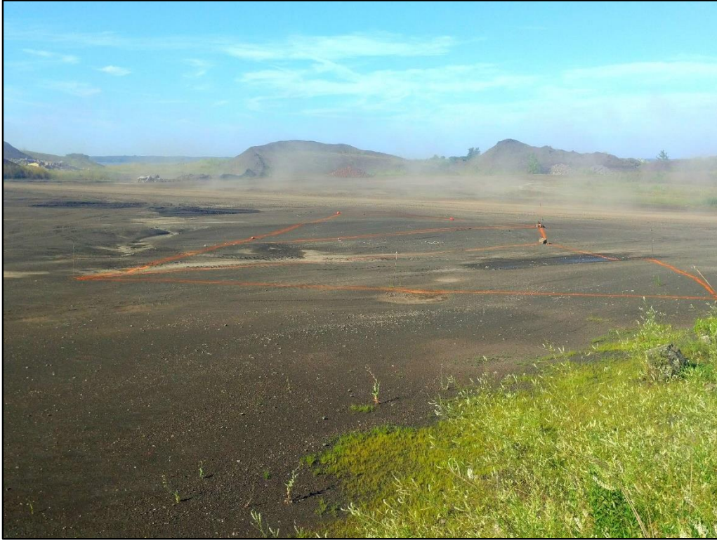
07/16/19-1: View to the south of the marked excavation boundary. The excavation is divided into a northern, southern, and middle section to facilitate stockpile management.
