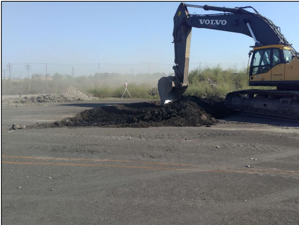
07/16/19-2: View to the north of the start of excavation at the B13-031 Response Area with a dust monitor present.
