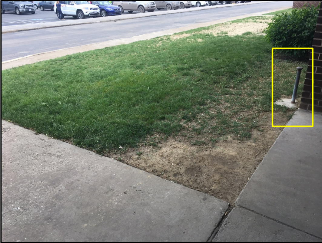
050317-1: “Vent pipe” (highlighted) and area of former Human Resources Building UST (near roadway), facing northwest.
