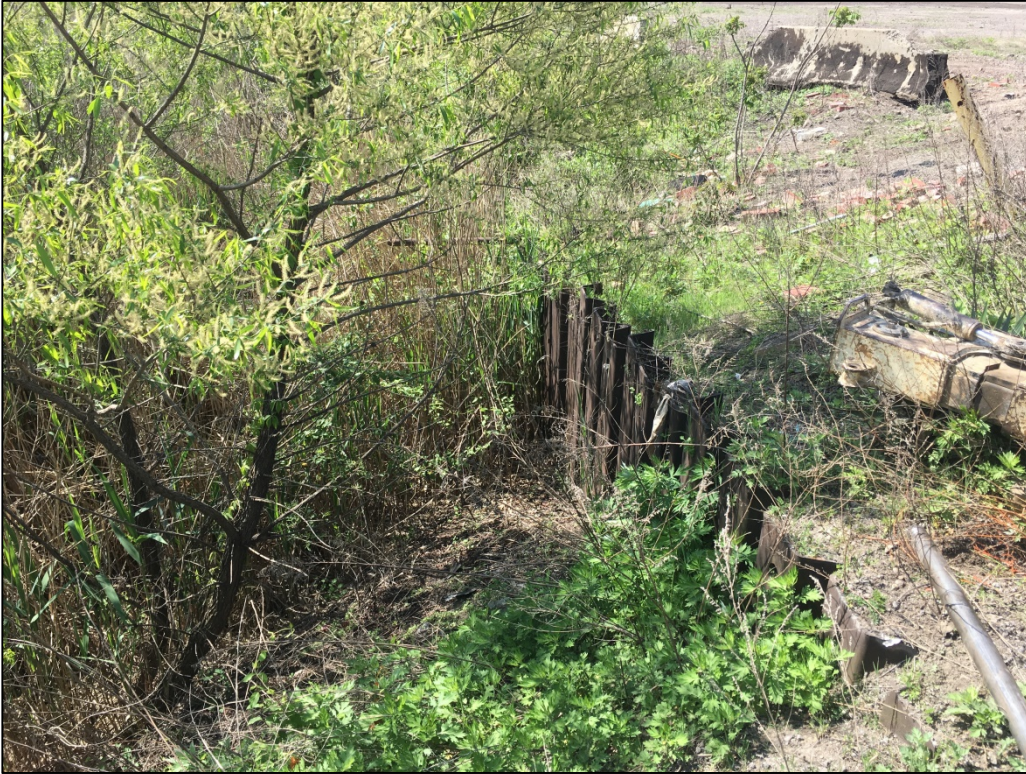
Photo 3: View of the sheet piling at the northern end of the PORI Lagoon.
