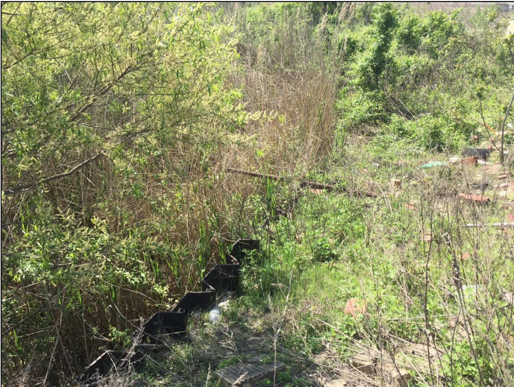
Photo 4: View of the sheet piling at the northern end of the PORI Lagoon.
