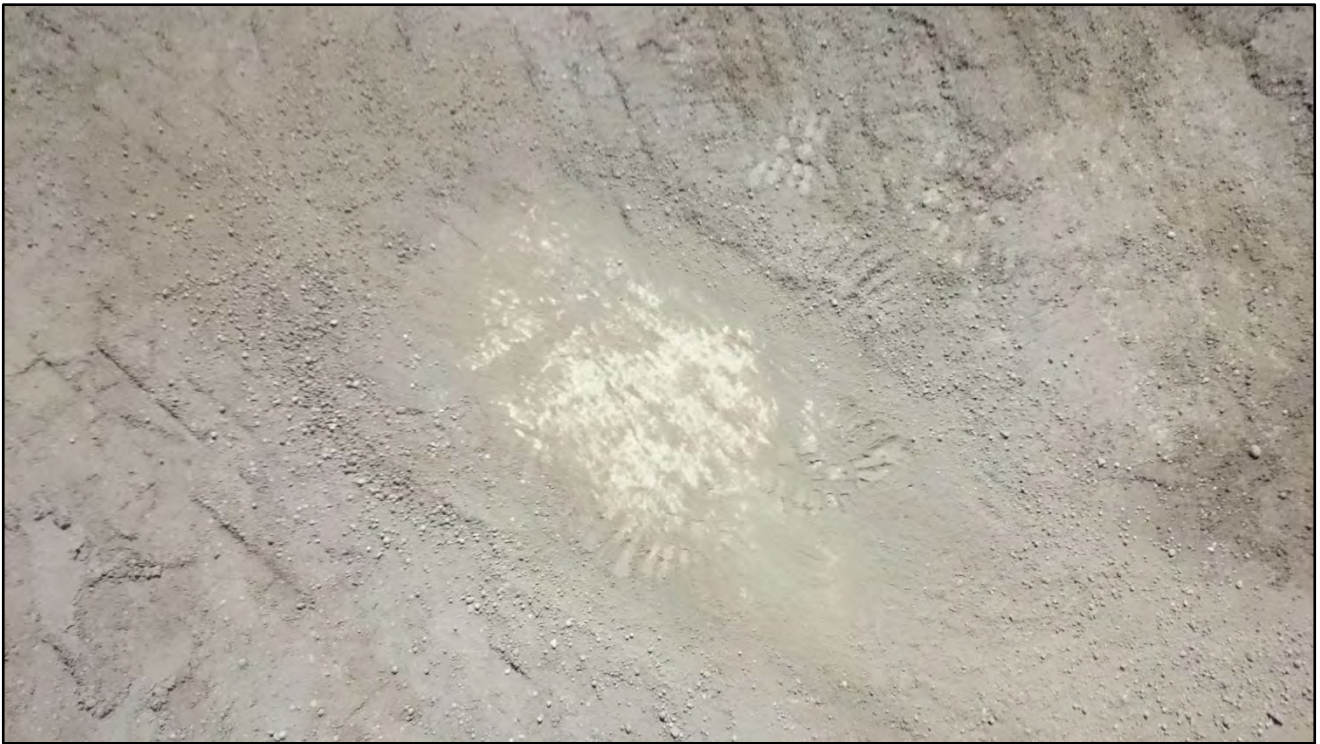
083116-10: Floor condition in north/central open area of the warehouse. Concrete floor mostly covered by thin dirt.
