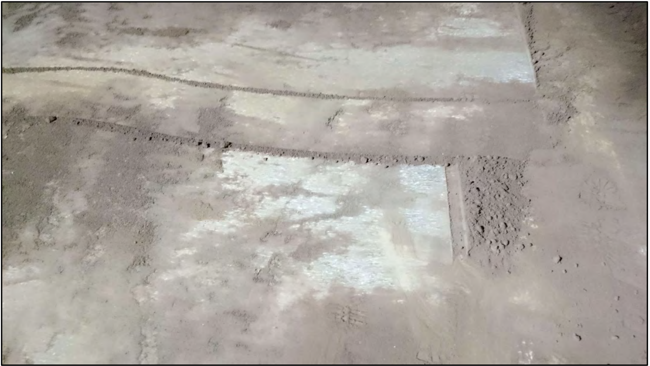
083116-9: Floor condition in northwest corner of the warehouse. Concrete floor mostly covered by thin dirt.
