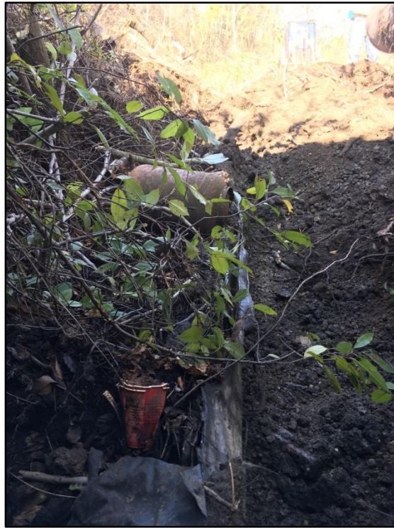
Photo 3: View of the sheet piling's southern extent and its alignment in the north direction.
