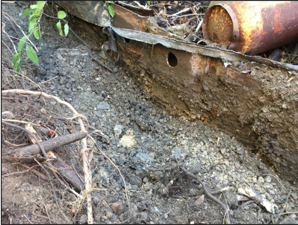
Photo 1: View of a section of the sheet piling (uncovered) located at the southern extent.
