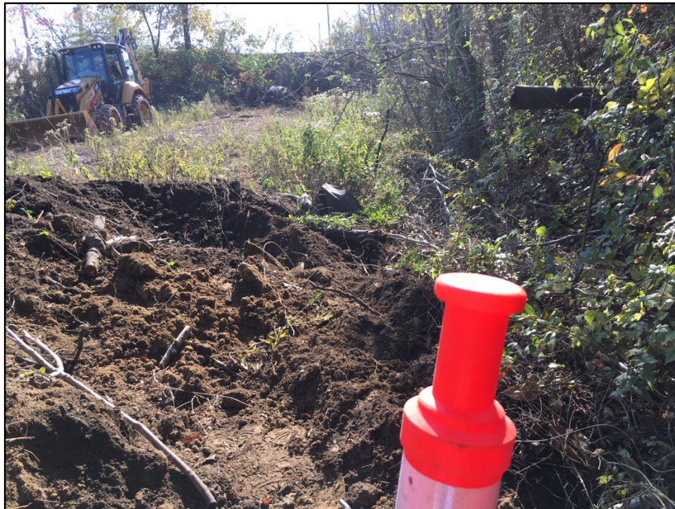
Photo 4: View of the sheet piling's northern extent and its alignment in the south direction.
