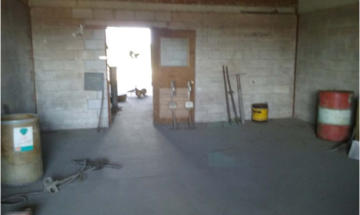
082616-7: Fourth room (furthest west and south) in the enclosed section of the Brick Shed . Picture facing north.
