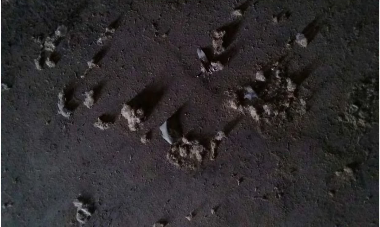
082616-3: Floor conditions within the enclosed area of the Brick Shed.
