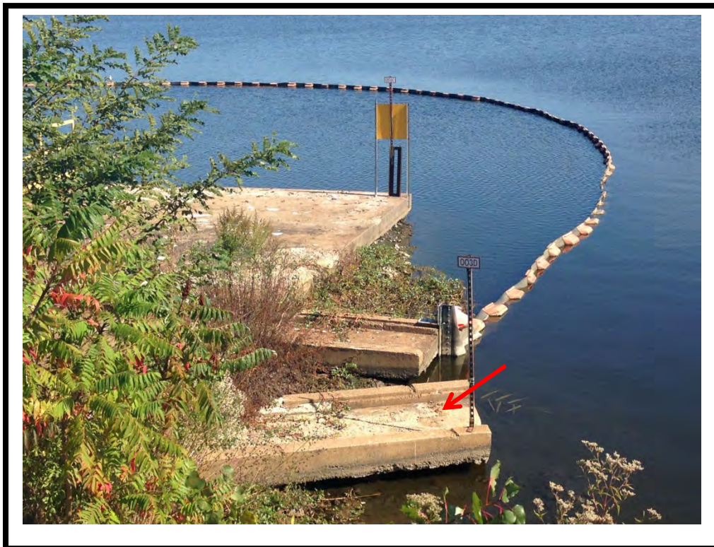
Photo 4: Looking northeast from shore towards end of culvert (the discharge point), baffle (boom), and concrete platform.
