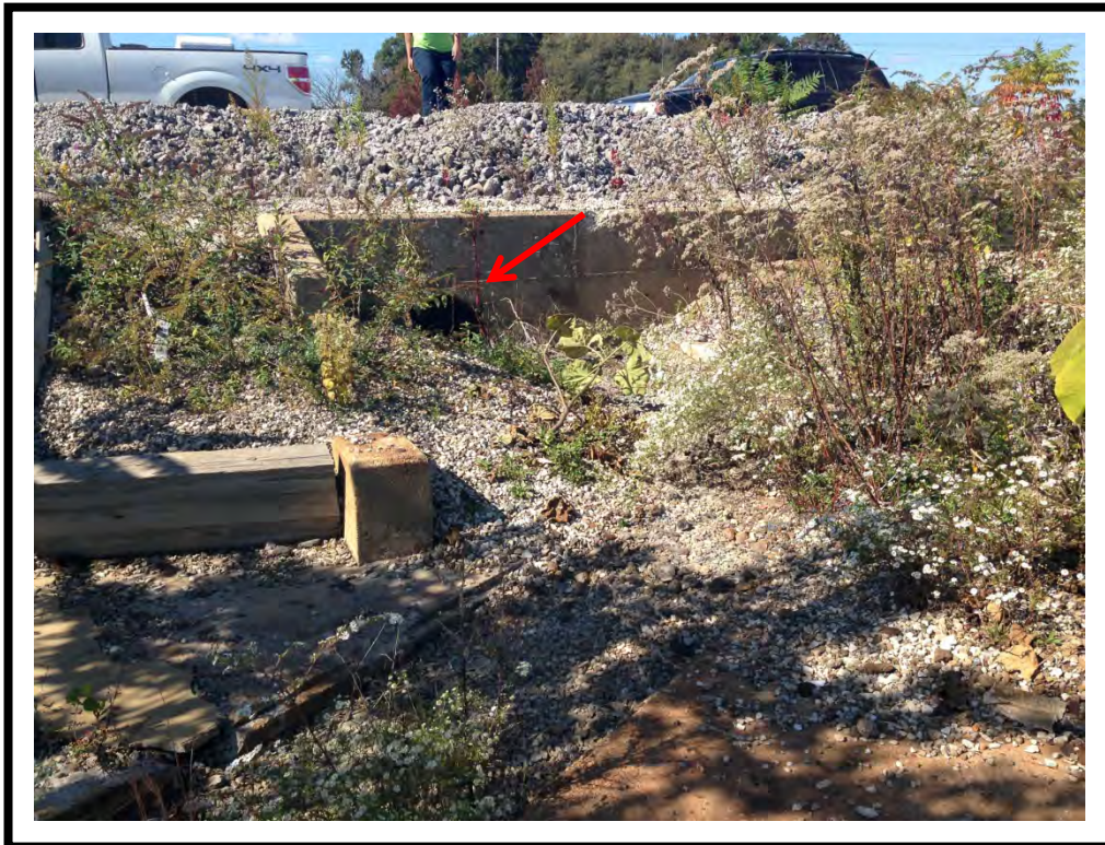
Photo 2: Looking west at headwall with outfall/drain pipe and shallow culvert filled with gravel.
