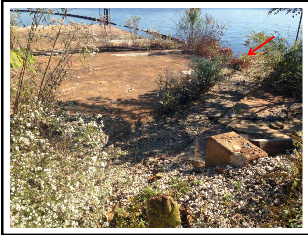
Photo 3: Looking southeast. Pipe discharges into shallow culvert filled with gravel prior to discharging to High Head Reservoir.
