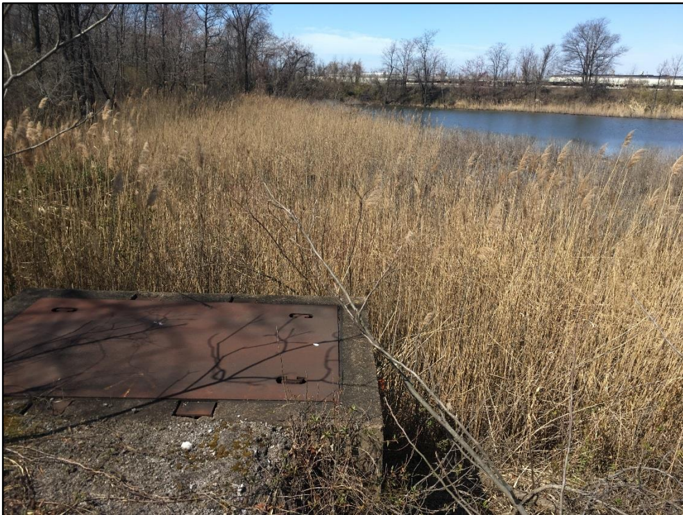
032819-4: Southern retention pond and stormwater structure at the southeastern boundary of the Site.
