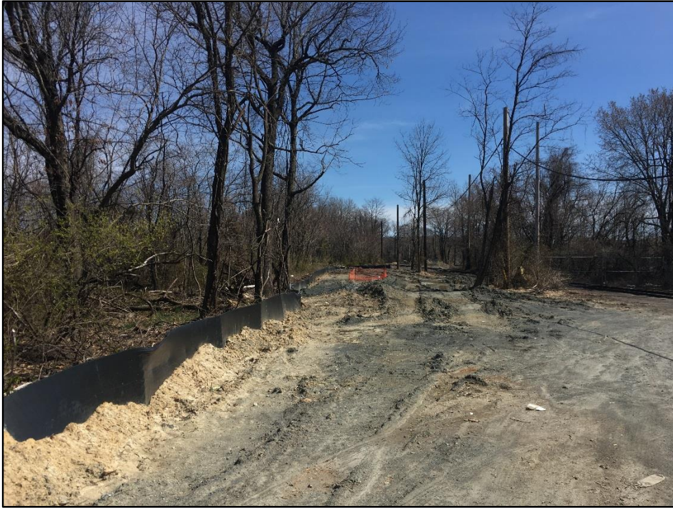
032819-5: A cleared area at the southern boundary of the Site. The area was cleared to allow for the installation of a sewer line.
