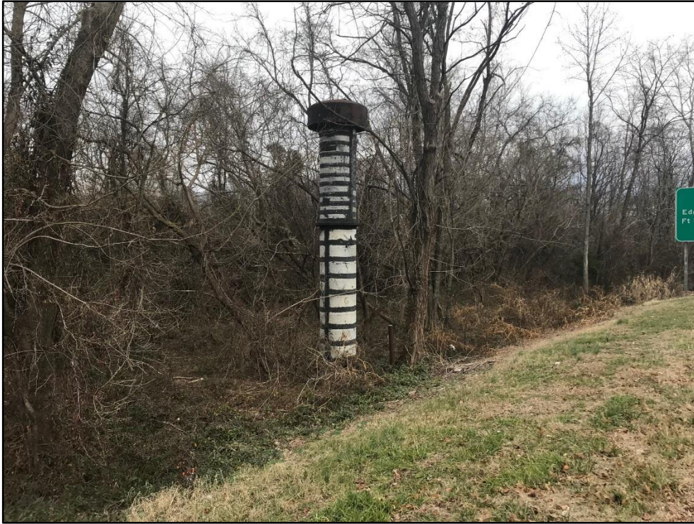
010719-9: An unknown ventilation pipe in the northeastern section of the Site. The pipe is in close proximity to the alignment of a 96-inch underground industrial water line.
