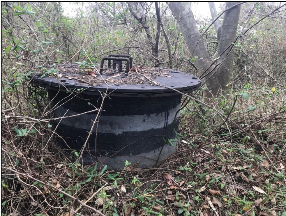
010719-10: An unknown manhole found in the Northeastern section of the Site. The manhole is in close proximity to the alignment of a 96-inch underground industrial water line.
