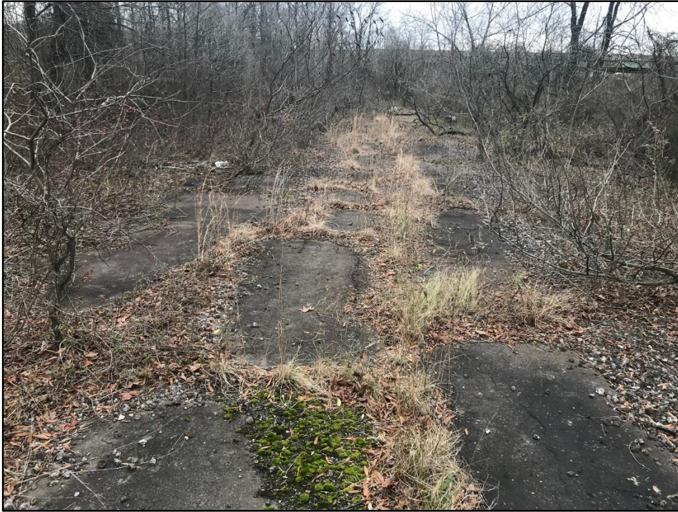
010719-1: View of concrete access road and wooded areas generally representative of conditions at the Site.
