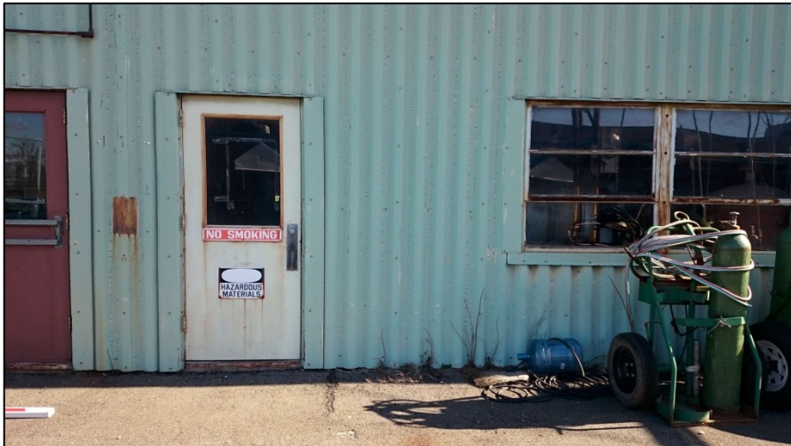
030216-8: Office & Hazardous Storage. Exterior view of boiler room (southern end) with hazardous label, facing northeast.
