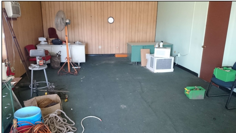
030216-5: Office & Hazardous Storage. Interior office room (northern end) with generic storage, facing northeast.
