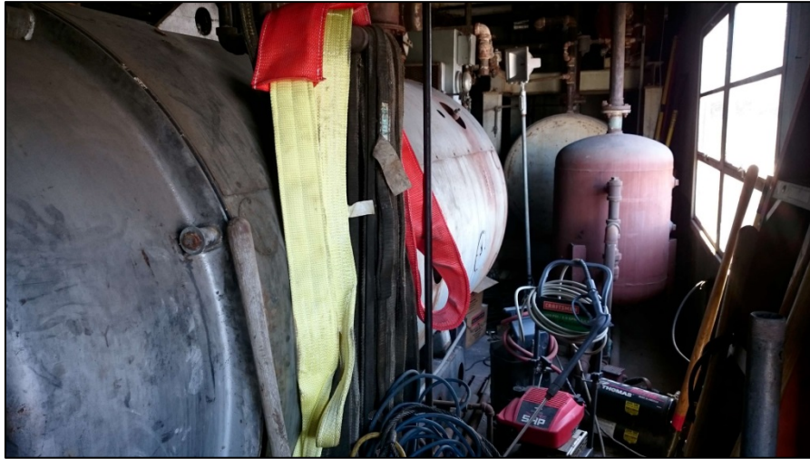
030216-10: Office & Hazardous Storage. View of boilers/steam pipes, facing southeast. No hazardous materials noted.
