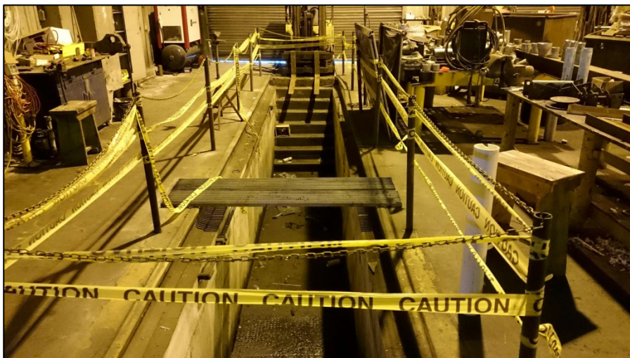
030216-21: Repair Shop. Interior view of western bay doors/rails with repair pit below floor level, facing north.
