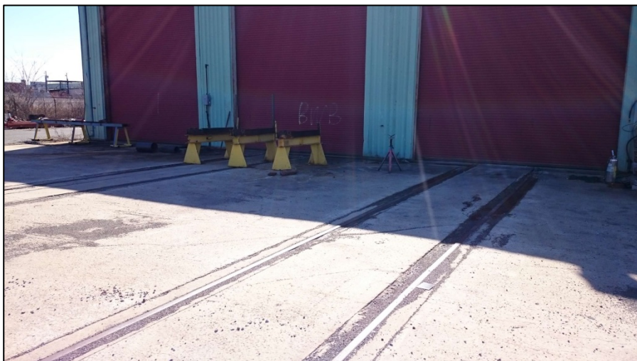
030216-15: Repair Shop. Exterior view of bay doors with rails (2 sets) leading into the shop, facing southeast.
