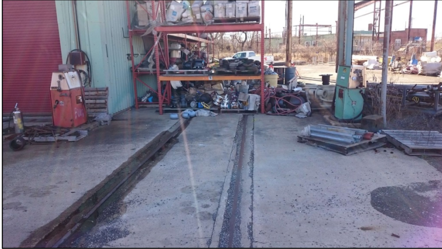
030216-13: Repair Shop. Exterior view of covered pad with generic storage, facing south. Noted location of fuel pumps.
