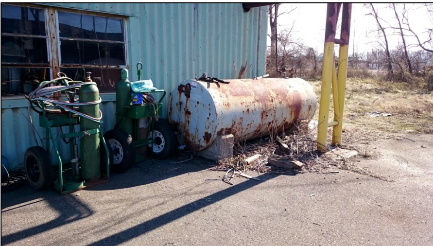
030216-9: Office & Hazardous Storage. Exterior view of boiler room fuel AST, facing east.
