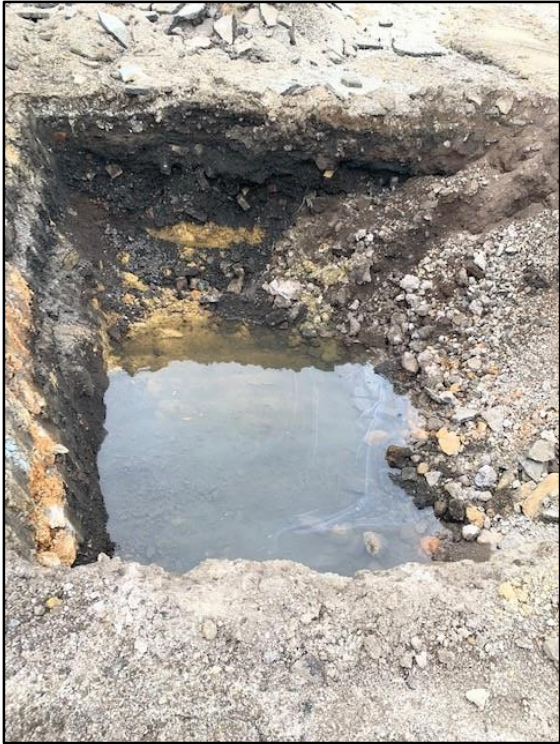
020520-1: Western test pit and standing surface water. MDE gave approval to backfill during their 2/20/2020 visit to the site.
