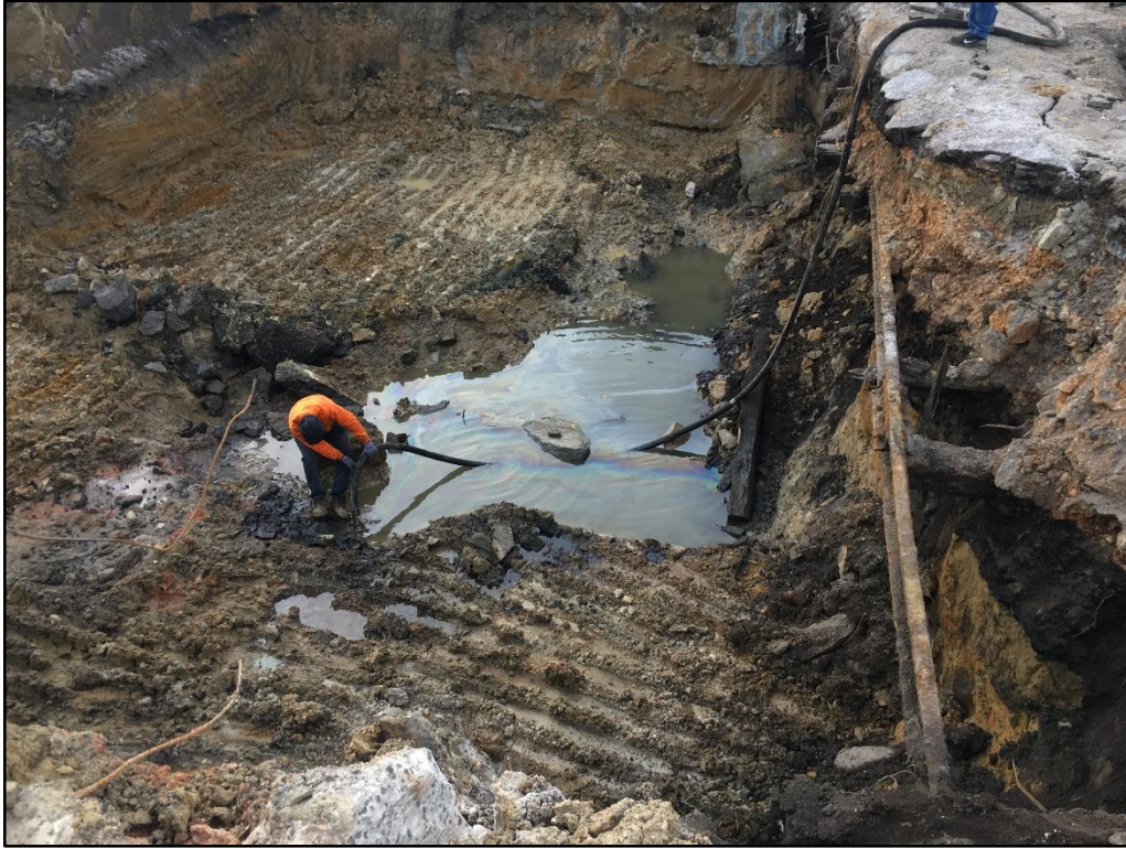
022020-1: Removal of surface water and NAPL from eastern test pit by ACE Environmental personnel.
