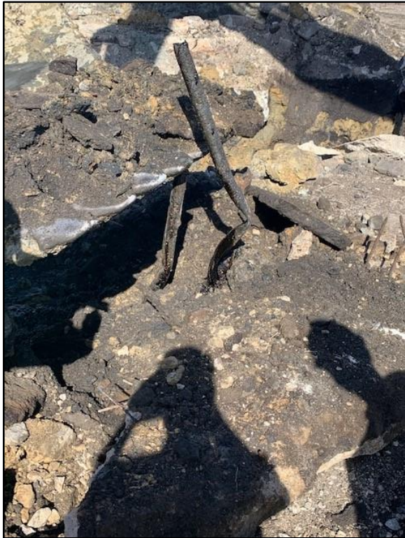
020320-4: An unknown pipe uncovered during the UST removal.
