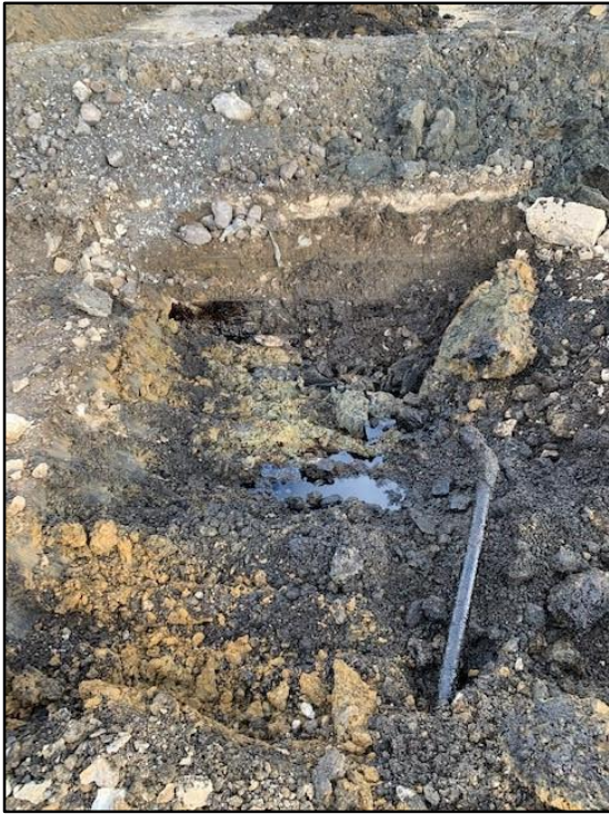
0120-1: Presence of NAPL during initial excavation in eastern test pit.
