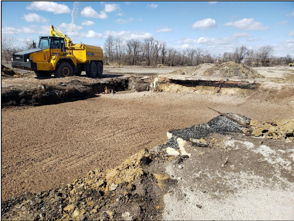
022720-2: Backfilling a few feet below the existing ground surface. Water was applied to some lifts as needed for material compaction.
