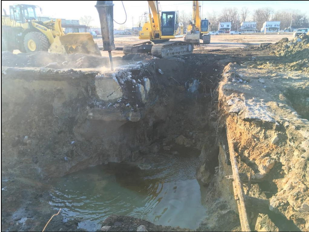
021720-1: An exposed rail and an additional subgrade structure encountered while expanding the eastern test pit excavation. The structure had been backfilled with soil and stone.
