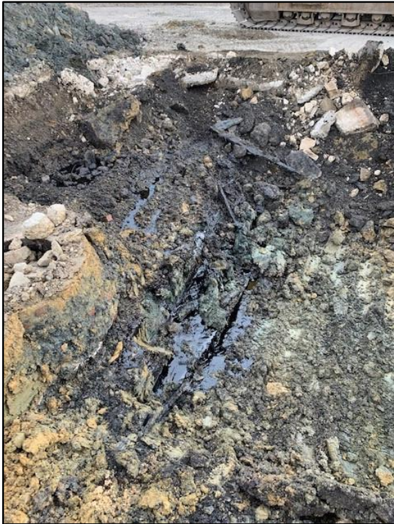
0120-2: Presence of NAPL during initial excavation in eastern test pit.
