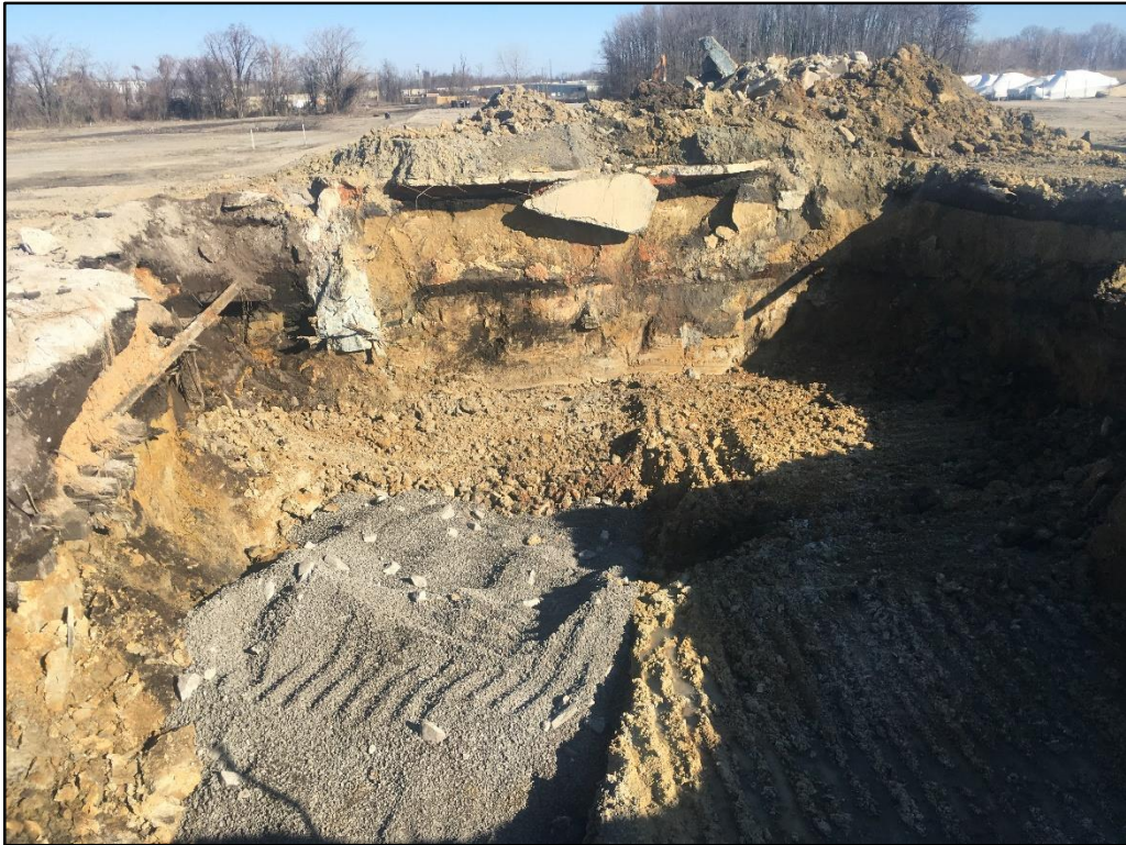
022120-1: Initial backfilling with #57 stone. The aggregate was used to partially backfill the excavation to above the groundwater level.
