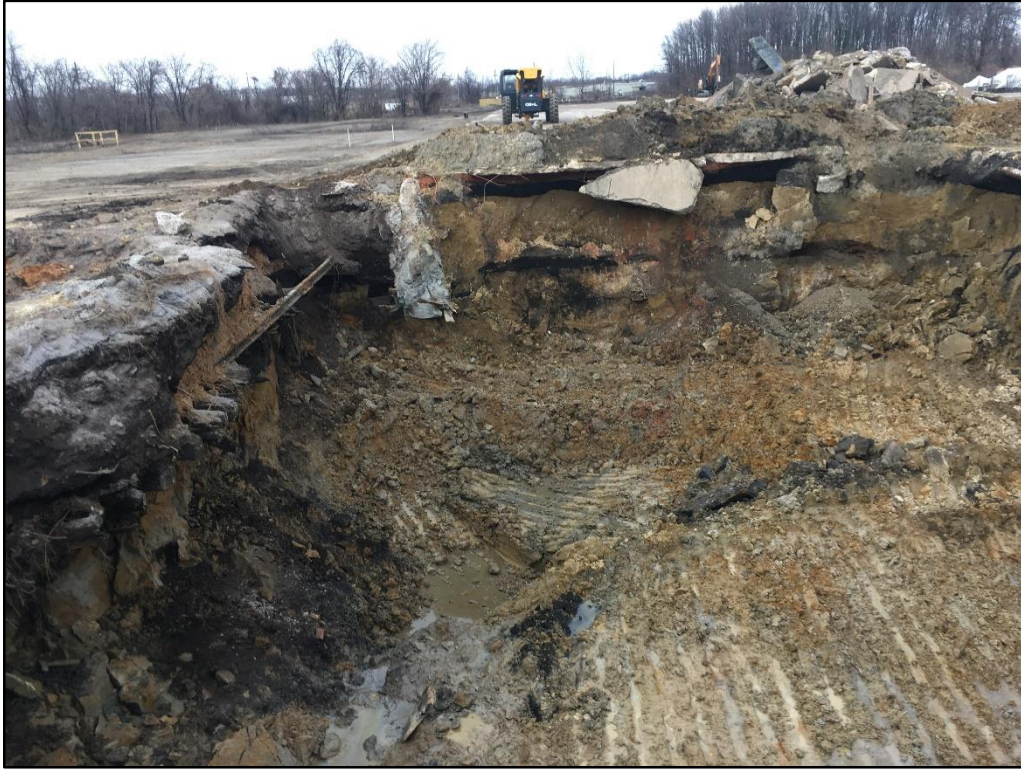
022020-3: View of the final eastern test pit excavation area from the southern sidewall.
