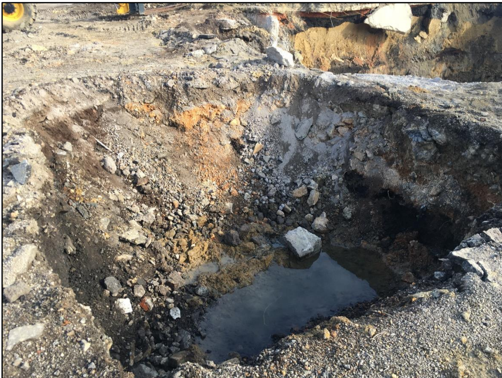
021820-2: A small volume of groundwater on the surface of the western test pit. The pit did not show signs of NAPL infiltration after two weeks of remaining open.
