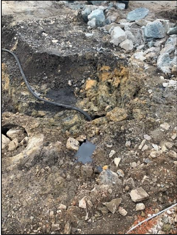
0120-3: Removal of material from buried underground storage tank (UST) during excavation using a vacuum truck.
