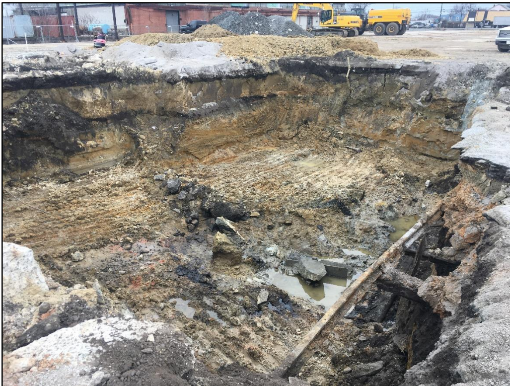
022020-4: View of the final eastern test pit excavation area from the northern sidewall.
