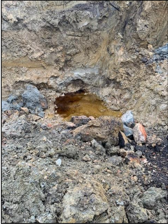
0120-5: Dark NAPL product at the surface of water in the excavated area.
