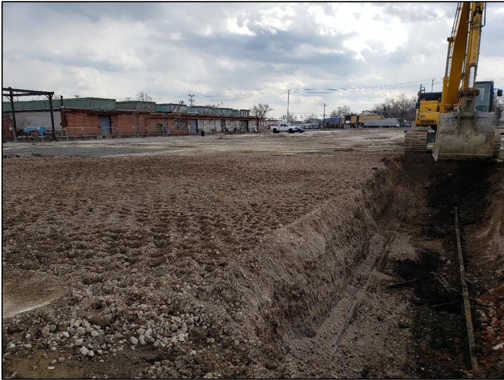
022820-1: Surface of the backfilled excavation. The rail lines were left exposed to be cut and removed in the future.
