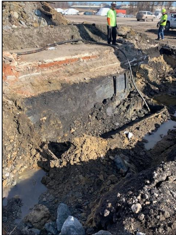
020320-3: ACE Environmental personnel removing NAPL product uncovered following UST removal using a vacuum truck.
