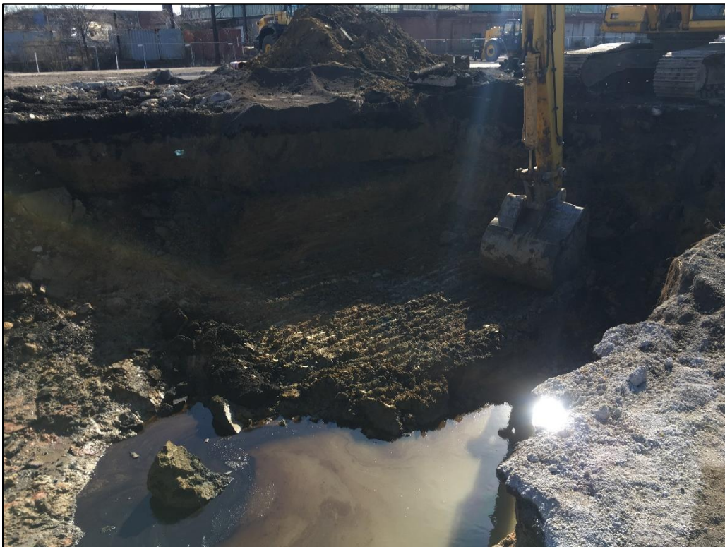
021720-2: Presence and removal of NAPL on the surface of water which infiltrated the eastern test pit excavation.
