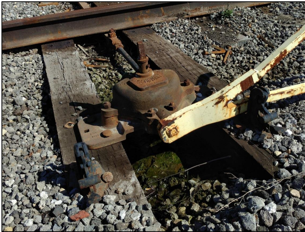
Photo 6 (3/27/19): Close-up view of railroad switch present along a section of existing track.
