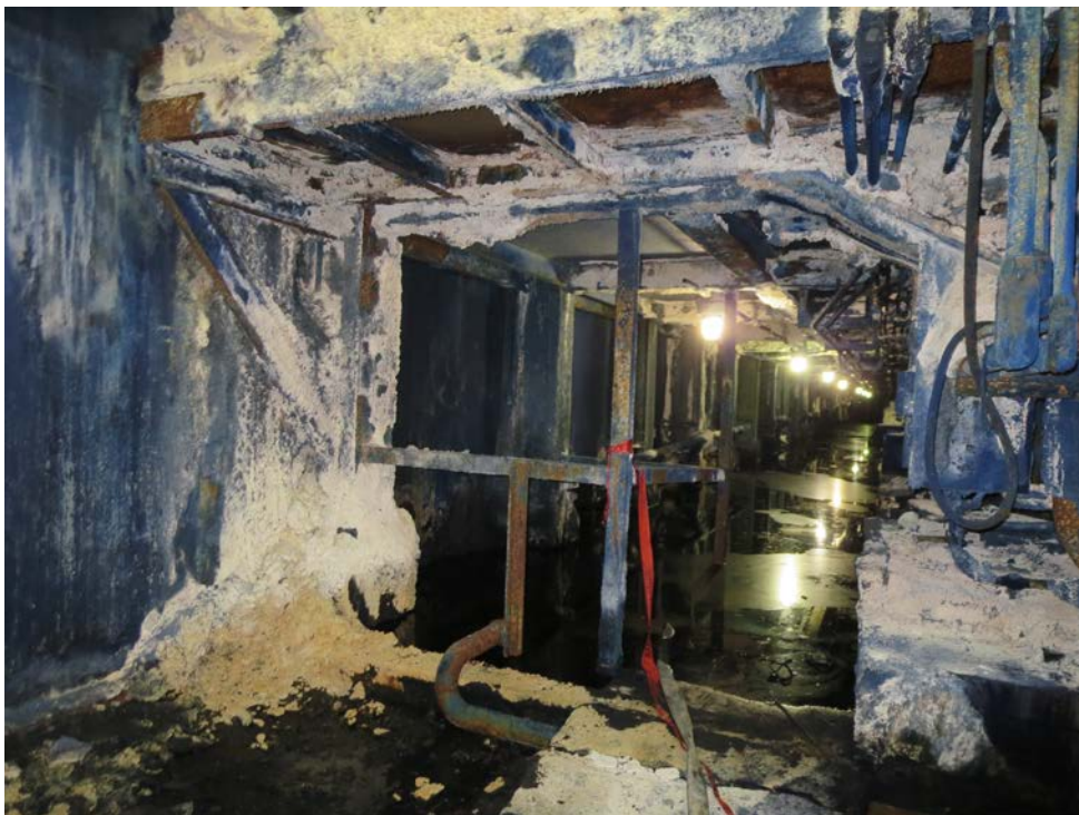
Photo 24: View of the Tin Mill basement with staining.
