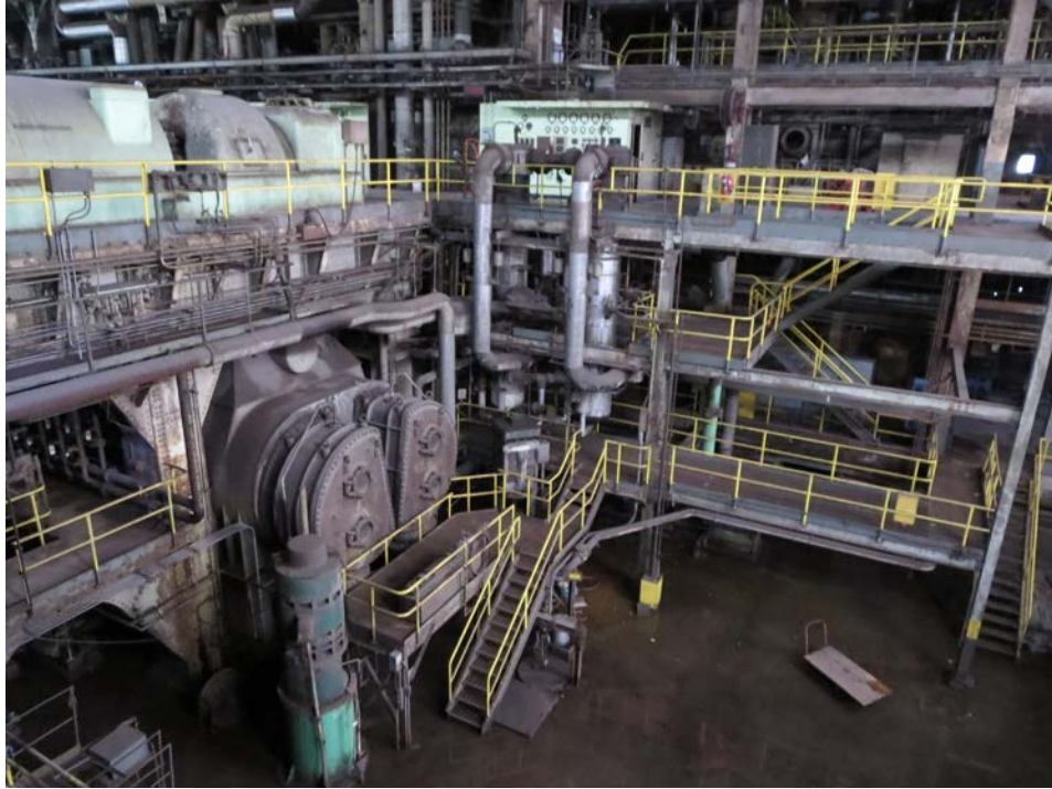
Photo 33: View of the "L" blast furnace interior flooding.
