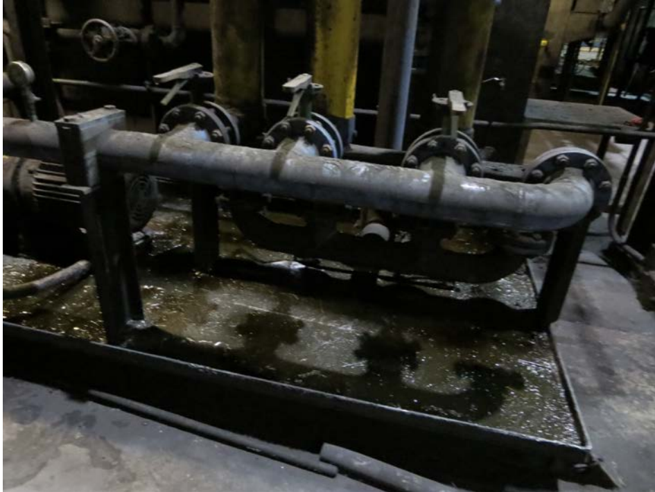
Photo 17: General view of staining in the Hot Strip Mill.
