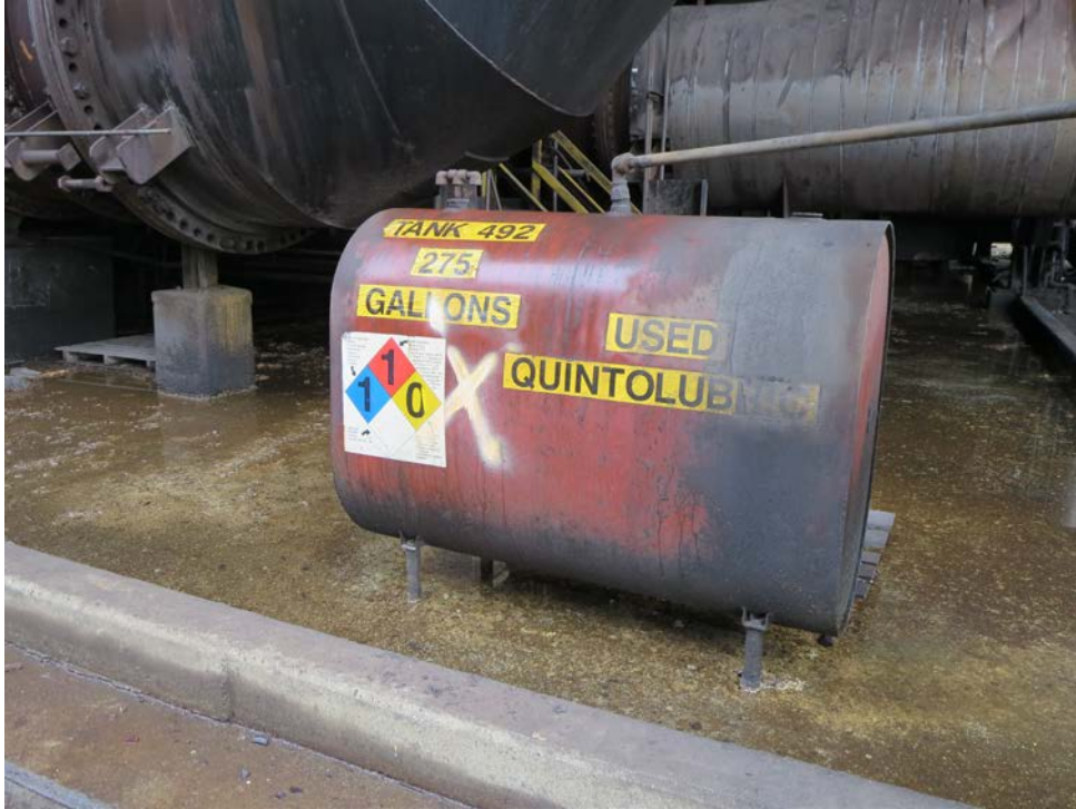
Photo 35: Representative view of in-use ASTs on the Property.
