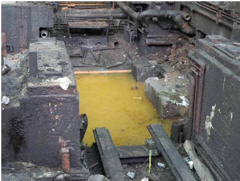
Photo 18: General view of staining in the Hot Strip Mill.
