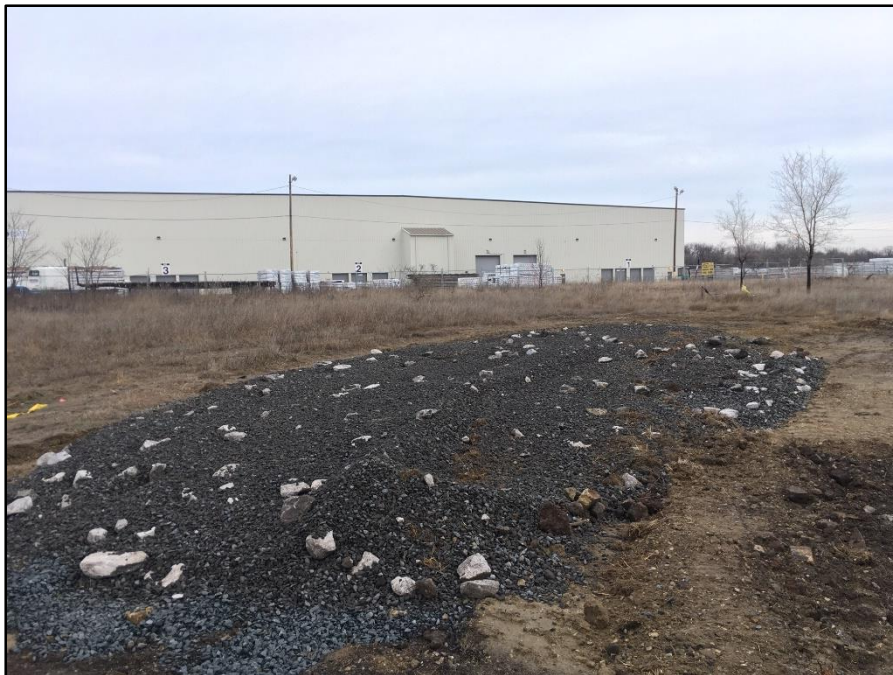
030620-1: View to the north of final backfilled state of A4-013 Response Area.
