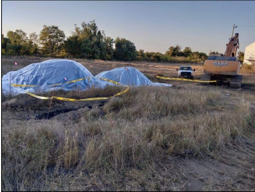
100419-5: View to the south of the completed A4 cadmium excavations and stockpiled soil.
