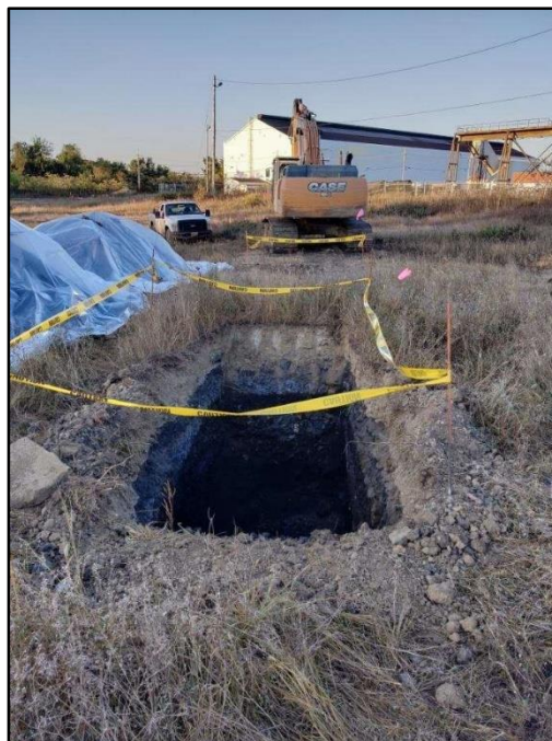
100419-4: View to the southwest of the completed northern excavation. Covered stockpiles are visible to the west of the excavation.
