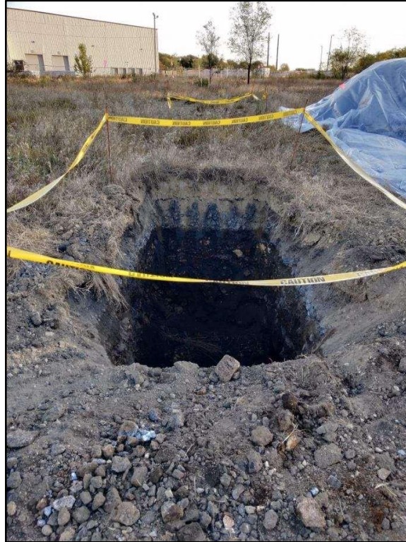
100419-3: View to the northeast of the completed southern excavation. Covered stockpiles are visible to the east of the excavation.
