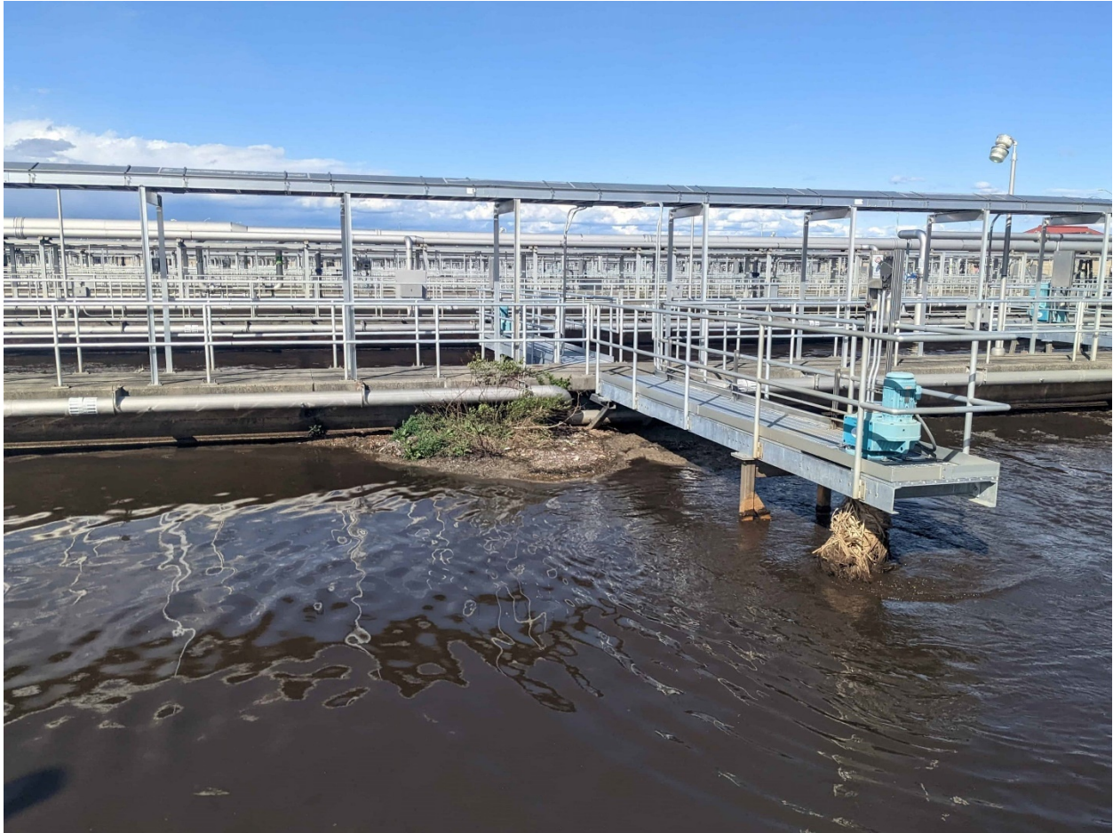
Activated Sludge Reactors
