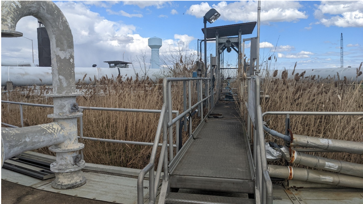
Gravity Sludge Thickener
