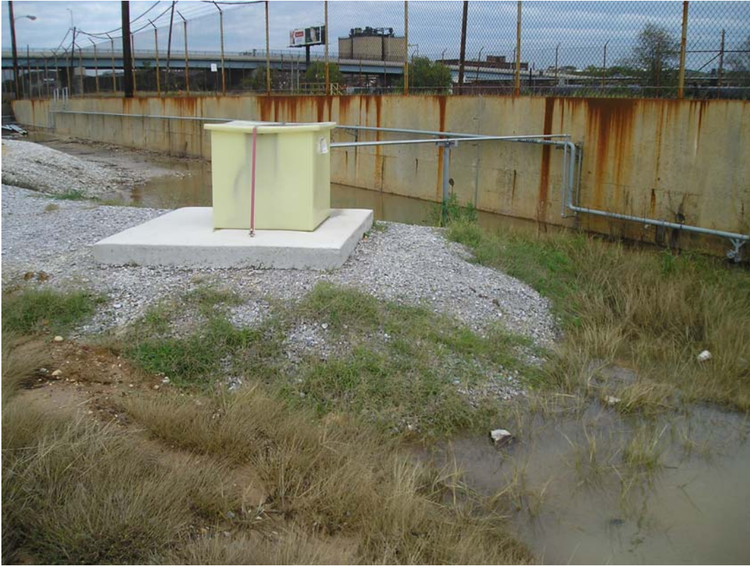
View of above grade sump in Toone Street Tankfield.
