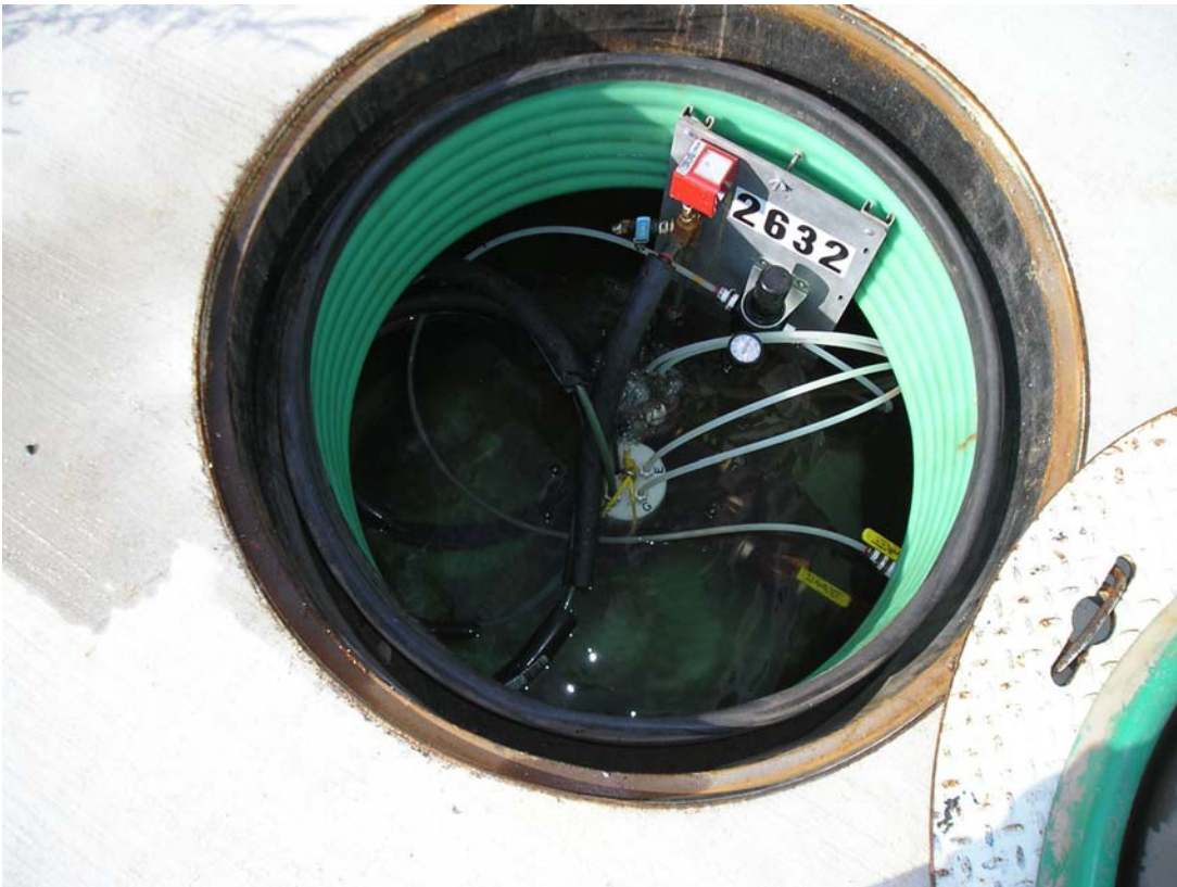
View of below grade sump in Main Terminal Area.
