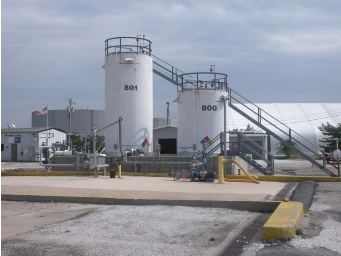
Main Terminal Area recovery tanks 800 and 801
