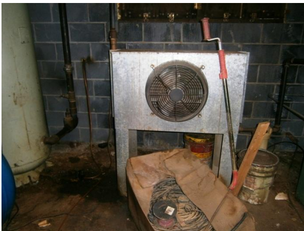
Photograph 17. Gear oil storage and minor oily staining in air compressor room of Furst Brothers building.
