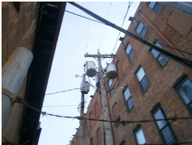
Photograph 5. Pole-mounted transformers located in the southern portion of the Site, along West Ostend Street.
