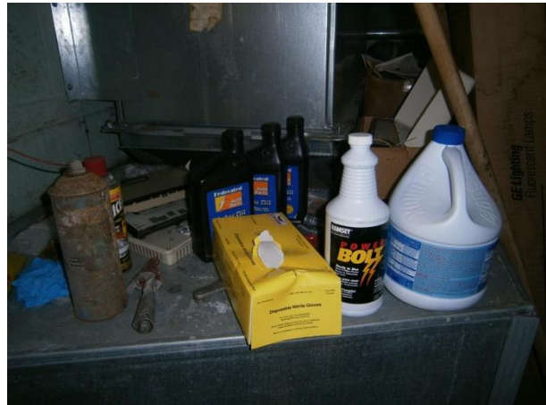
Photograph 52. Routine maintenance supplies in boiler room located in the northern portion of the US Post Office building.
