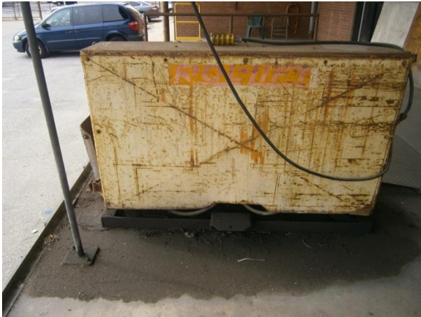
Photograph 47. Oily staining beneath aboveground hydraulic lift located on the loading dock.
