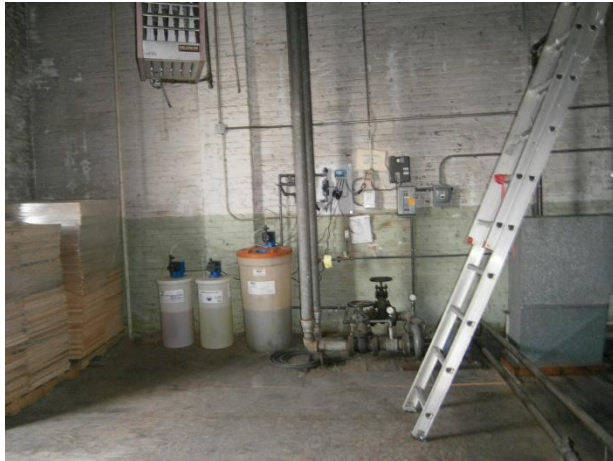
Photograph 41. Water softener drums in fourth floor of southern VacPac building.
