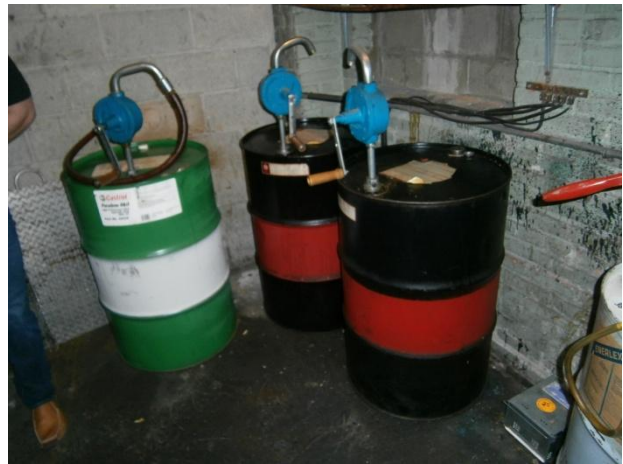
Photograph 32. Hydraulic oil drums in northwestern portion of the air compressor room.
