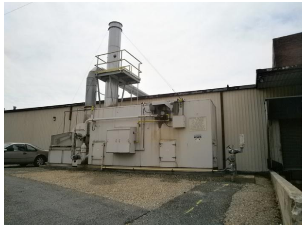
Photograph 26. Air scrubber/oxidizer along northern portion of the northern VacPac building.
