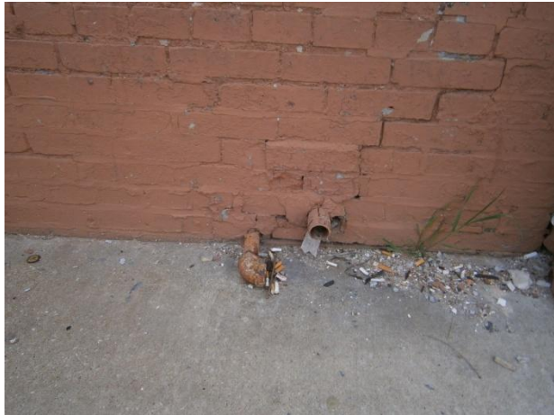
Photograph 7. Unknown pipe along western portion of the Furst Brothers building.
