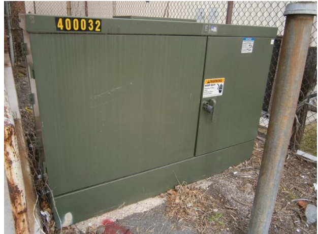
Photograph 48. Pad-mounted transformer located along northern portion of the US Post Office building.
