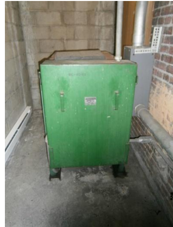
Photograph 36. Hydraulic reservoir in elevator mechanical room located behind the freight elevator.
