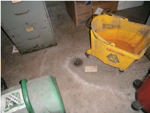
Photograph 51. Floor drain in boiler room located in the northern portion of the US Post Office building.
