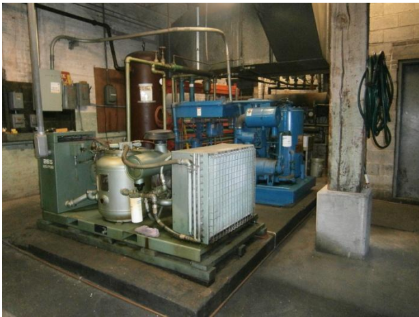
Photograph 31. First floor air compressor room in the northern portion of the southern VacPac building.
