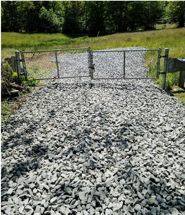
Photo 4. View of the completed SCE at the site gate, looking toward the southwest.
