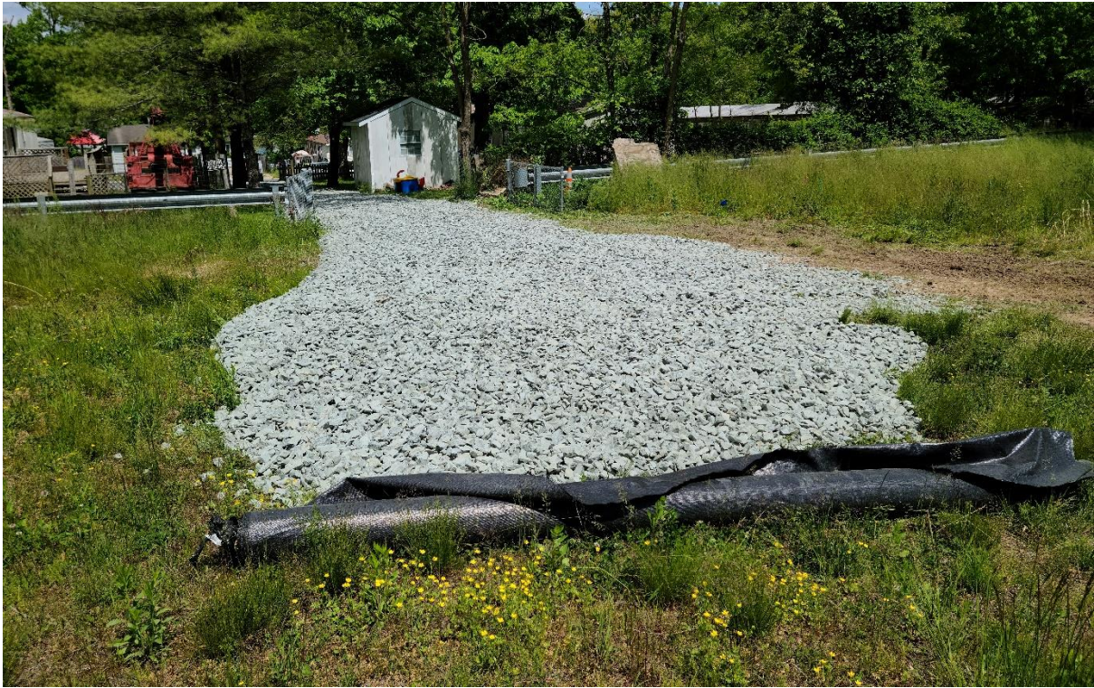
Photo 3. View of the nearly completed SCE from its on-site end, looking toward the northeast.
