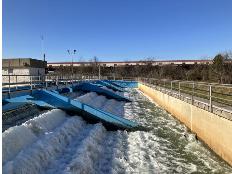
Image 03: Step Aeration system, final effluent.
