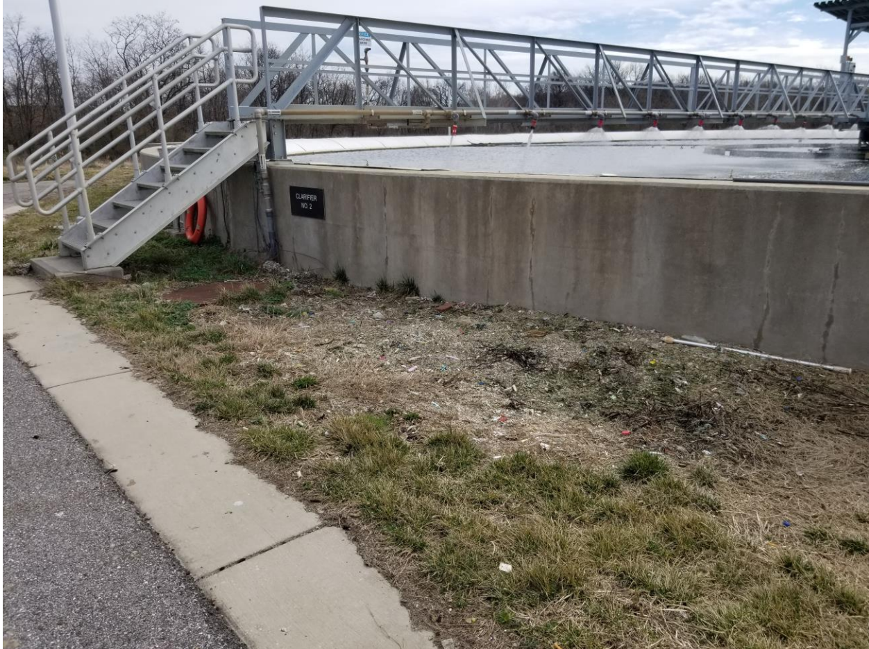
2/24/23 Solids and trash on the ground next to backwash clarifier #2.
