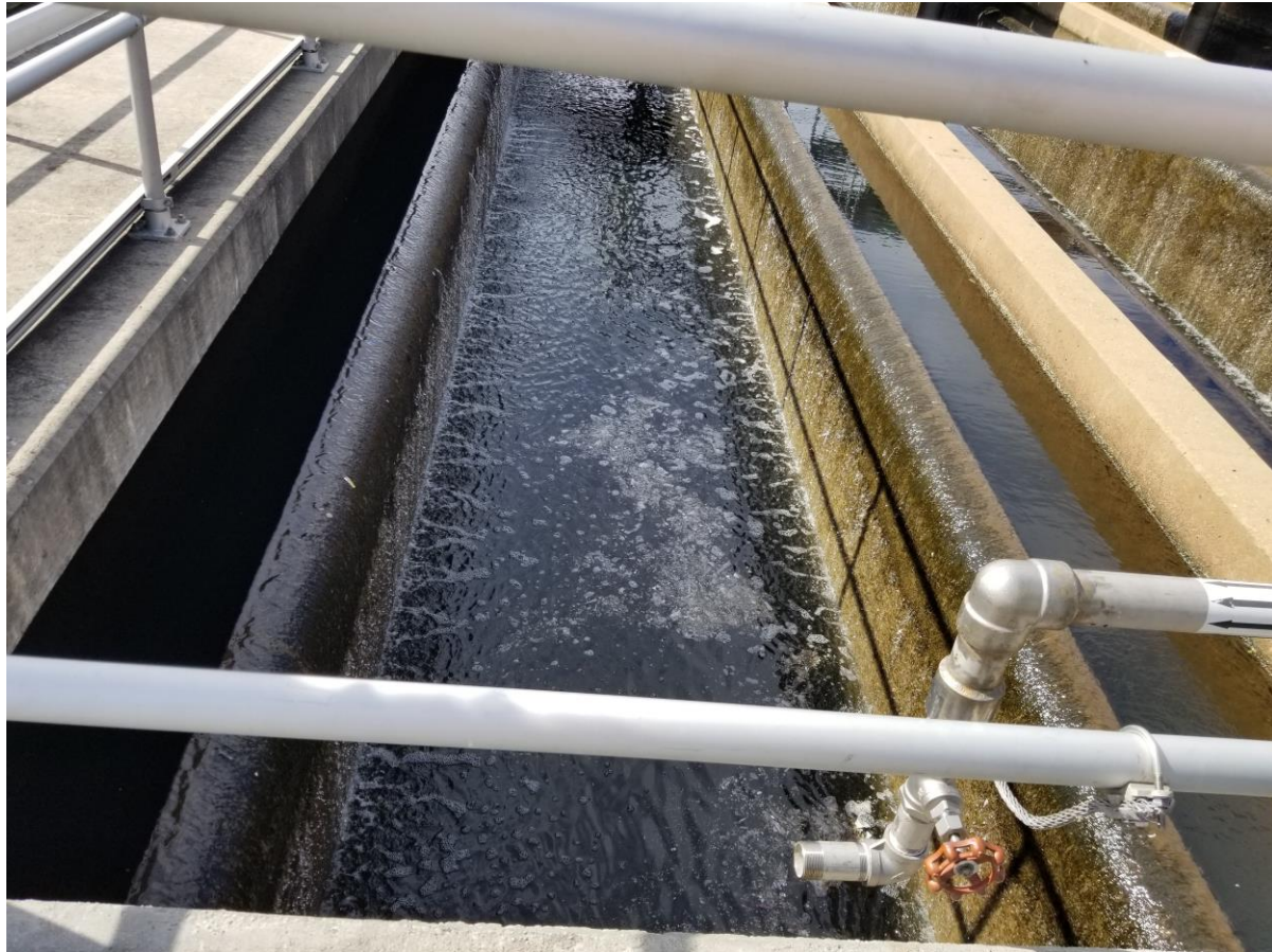
2/24/23 Solids and trash floating on water surface in the DNFs.
