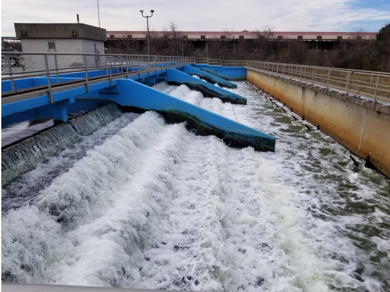
2/24/23 Final Effluent at the step aeration system.
