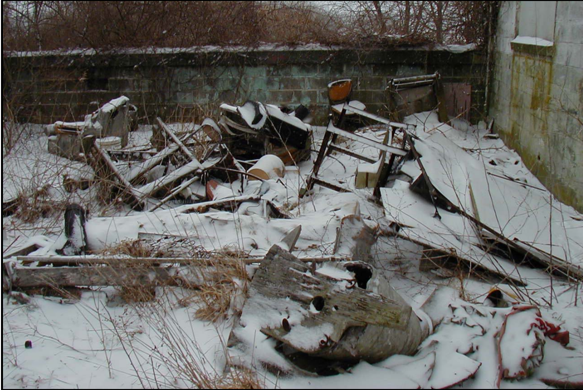
Photograph of debris pile on north end of the masonry building.
