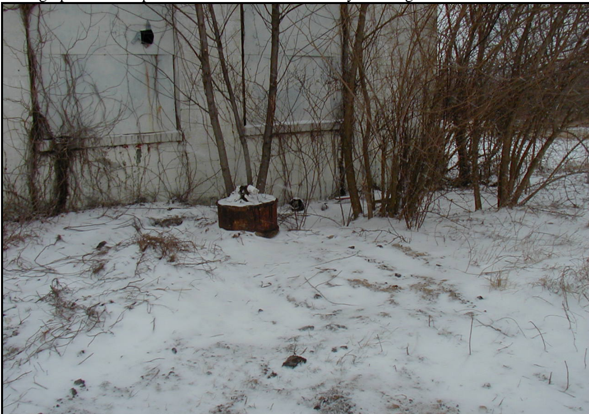
Photograph of the 10,000 gallon UST intake valve located on the south side of the building.
