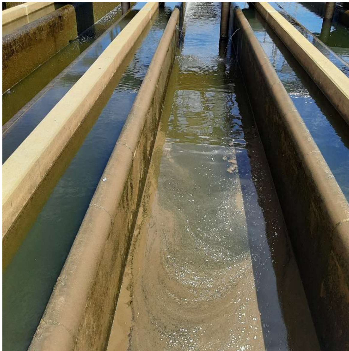
8/16/22 Solids in filter located in Quad 3. This should be investigated.
