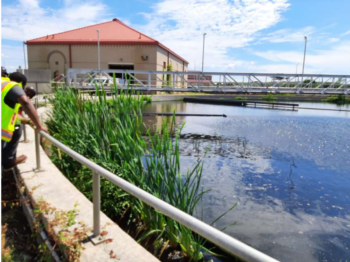
8/16/22 Secondary clarifier #5A. Reed grass growing on and around the weirs.
