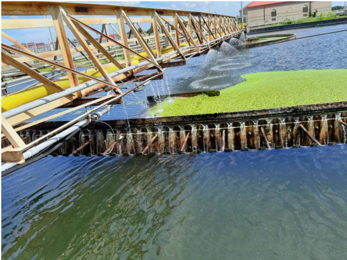
8/16/22 Secondary clarifier 13A. Opening to the scum pit is clogged. Water spray is being used to try to keep the pit open.
