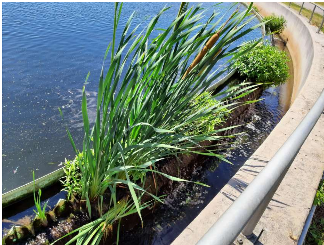
8/16/22 Vegetation on the weir of a secondary clarifier
