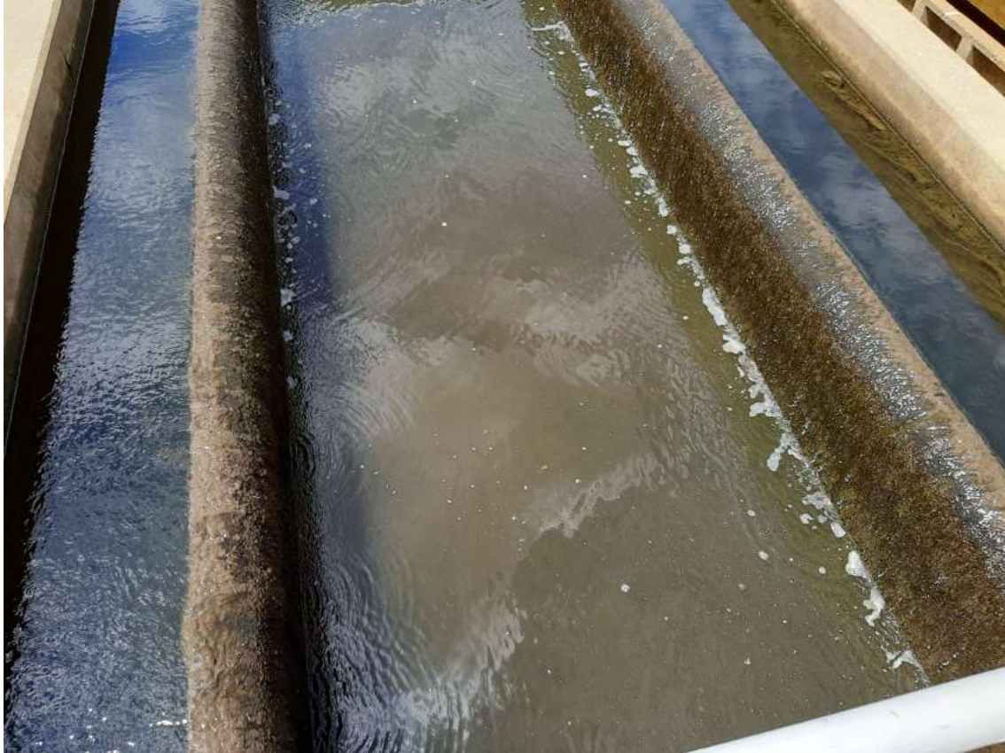
8/16/22 DNF in Quad #3 Note dark grey water showing high solids concentration
