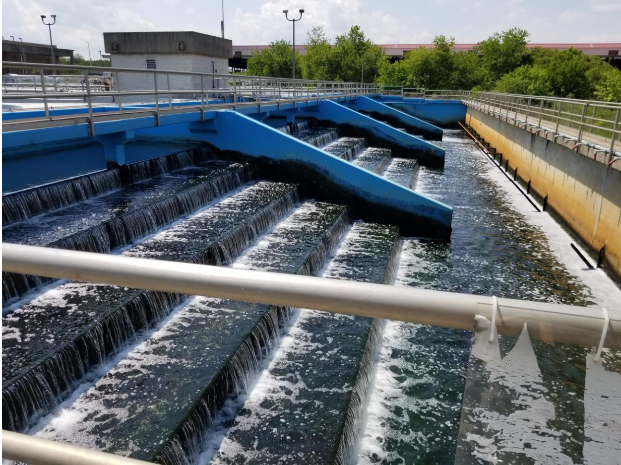
4/26/23 Final Effluent at the step aeration system.
