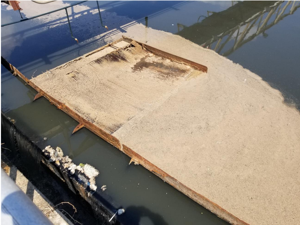
4/26/23 PST #1 – scum trough was observed to be clogged with scum.
