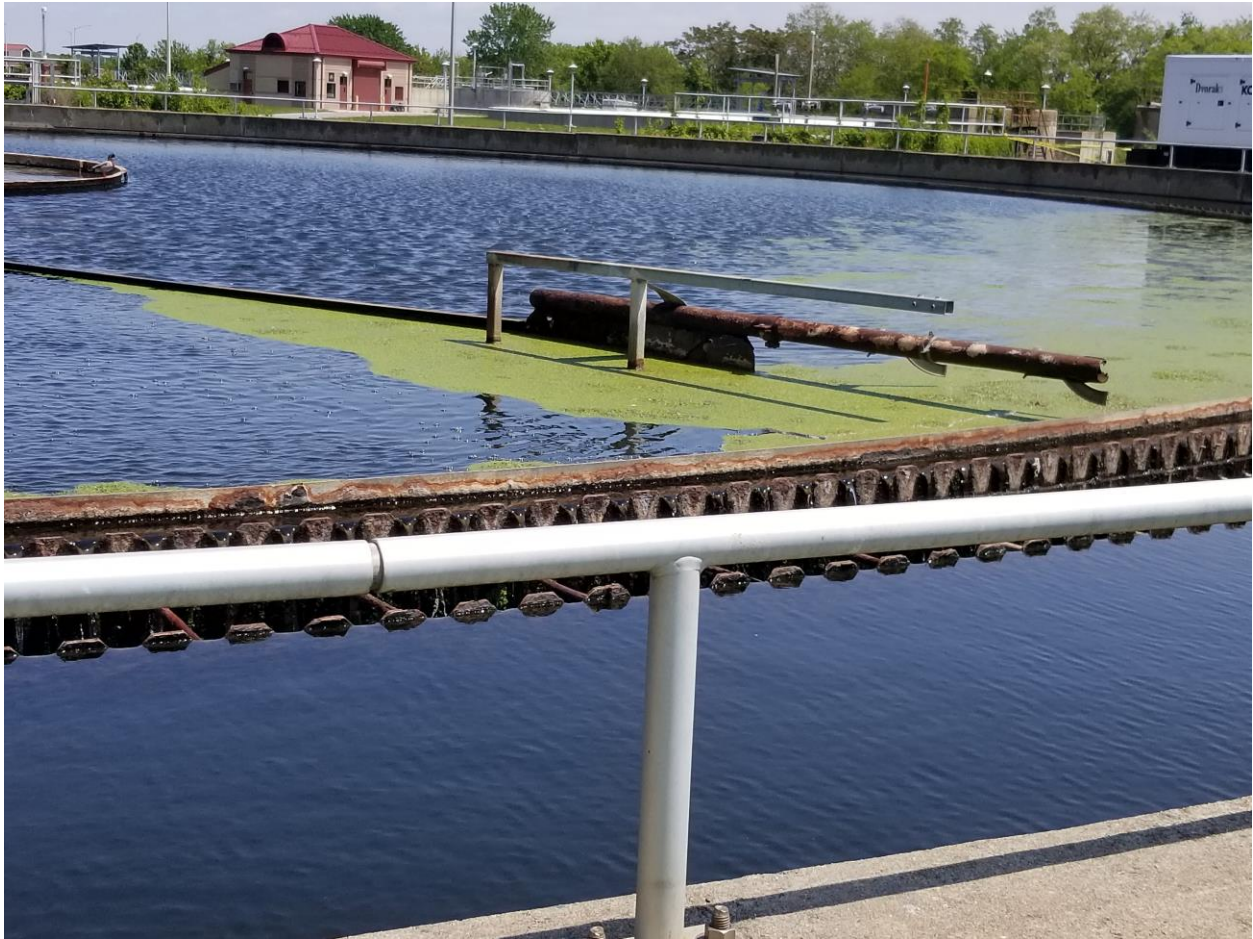
4/26/23 Secondary clarifier 12A – the skimming arm on secondary clarifier 12A was observed to be missing the skimming flap.
