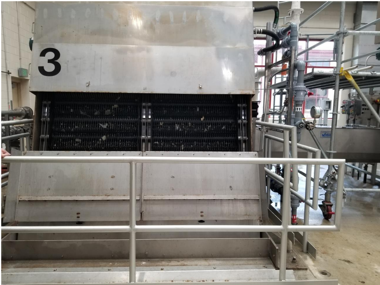
4/26/23 Fine screening unit #3 was observed to be operating during inspection.
