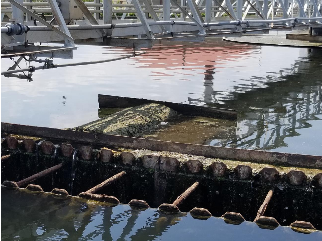
4/26/23 Secondary clarifier 14B – scum trough was observed to be clogged with scum.
