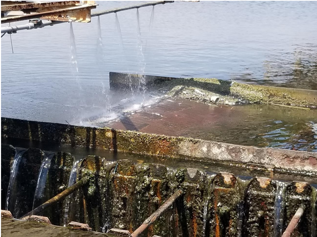
4/26/23 Secondary clarifier 13B – scum trough was observed to be clogged with scum.
