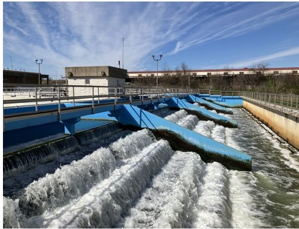
Image 02: Step Aeration system, final effluent.
