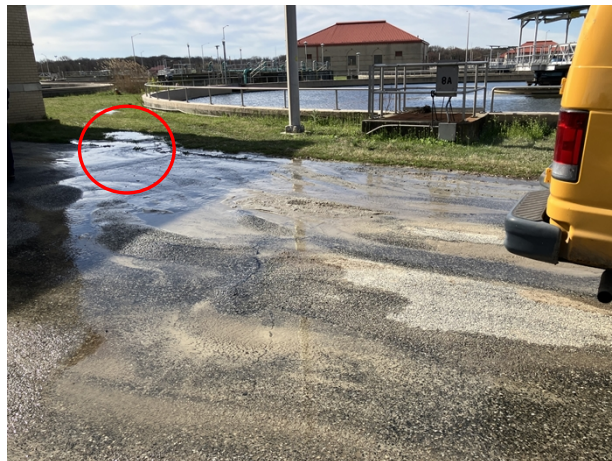
Image 06: Potable water leak. Location of leak circled in red.
